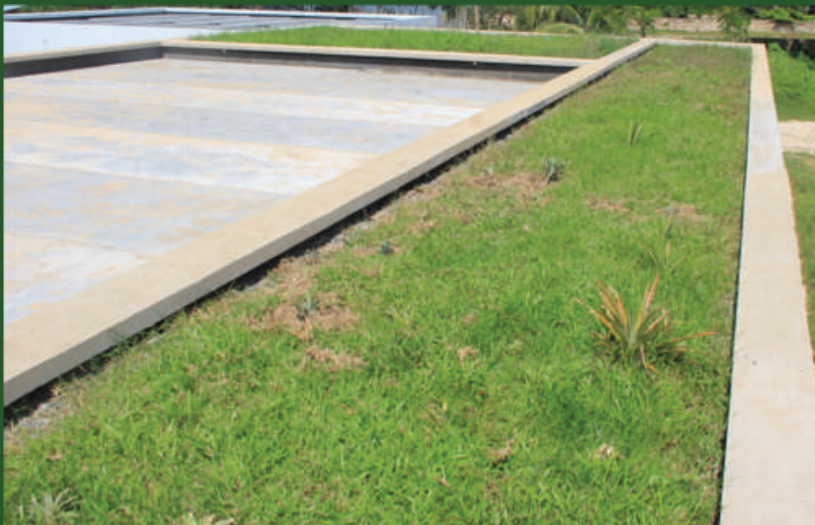
Figure 3.5 Pineapple green roof at Knai Bang Chatt
