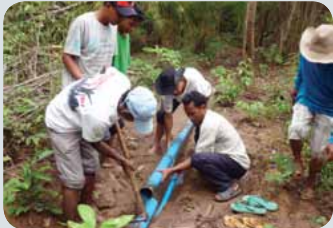
Villagers install pipe to bring clean water from a nearby waterfall into villagers' homes in Kampong Speu province. Photo: Mlub Baitong
