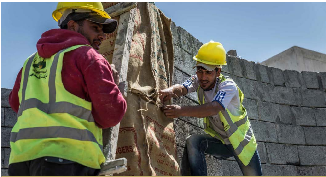
SIGNIFICANT PROGRESS WAS MADE ON THE REHABILITATION OF THE ABI TAMMAM POLICE STATION, WHERE MASONRY WORK AND CASTING OF CONCRETE WAS UNDERTAKEN. ©UNDP IRAQ/CLAIRE THOMAS
