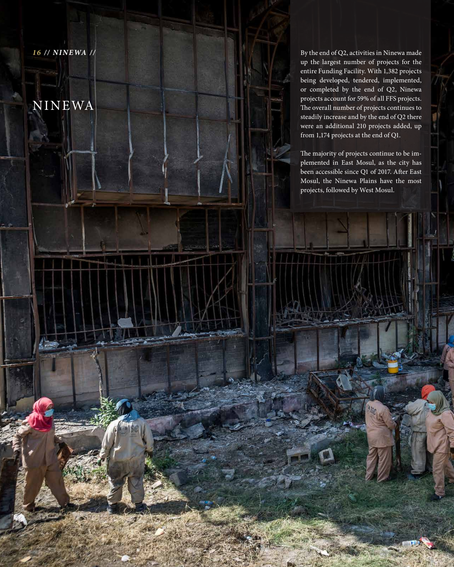
MEMBERS OF A FFS SUPPORT CASH FOR WORK TEAM, WORKING TO CLEAR RUBBLE AND DEBRIS FROM AROUND THE CENTRAL LIBRARY AT THE UNIVERSITY OF MOSUL IN EAST MOSUL. ©UNDP IRAQ/CLAIRE THOMAS
