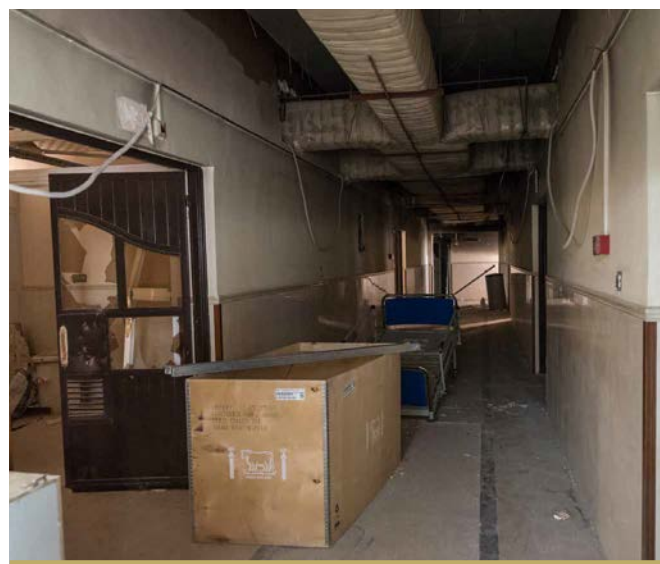
A DAMAGED COORIDOR IN HAMDANIYA HOSPITAL. THE NEXT PHASES OF WORK ON THE HAMDANIYA HOSPITAL ARE WAITING ONLY APPROVAL OF THE BOQS, AND ADDITIONAL WORKS TO IMPROVE MEDICAL EQUIPMENT IS UNDERWAY. ONCE TOTALLY COMPLETED, THE HOSPITAL IS ABLE TO SERVICE A POPULATION OF 500,000 BENEFICIARIES. ©UNDP IRAQ/CLAIRE THOMAS.
