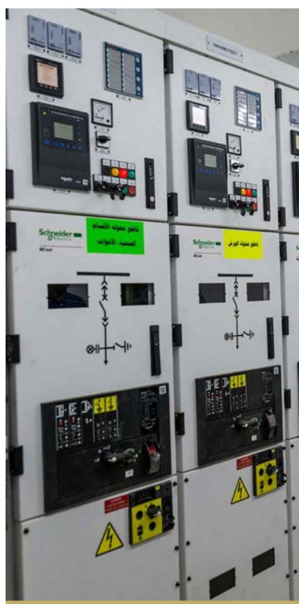
NEW SWITCHGEAR AT THE NORTHERN TECHNICAL UNIVERSITY IN EAST MOSUL. THE RESTORATION OF THE ELECTRICAL NETWORK OF THE UNIVERSITY WAS COMPLETED DURING THE REPORTING PERIOD. ©UNDP IRAQ/CLAIRE THOMAS
