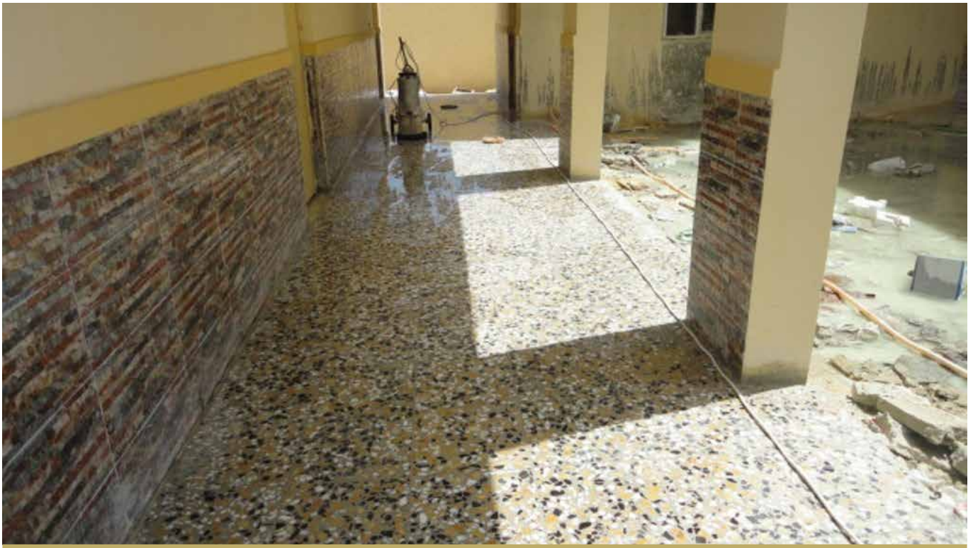
WORK PROGRESSED WELL ON THE AL-NOBOUGH SECONDARY SCHOOL IN FALLUJAH, WHICH REACHED 98% COMPLETION BY THE END OF THE REPORTING PERIOD.
