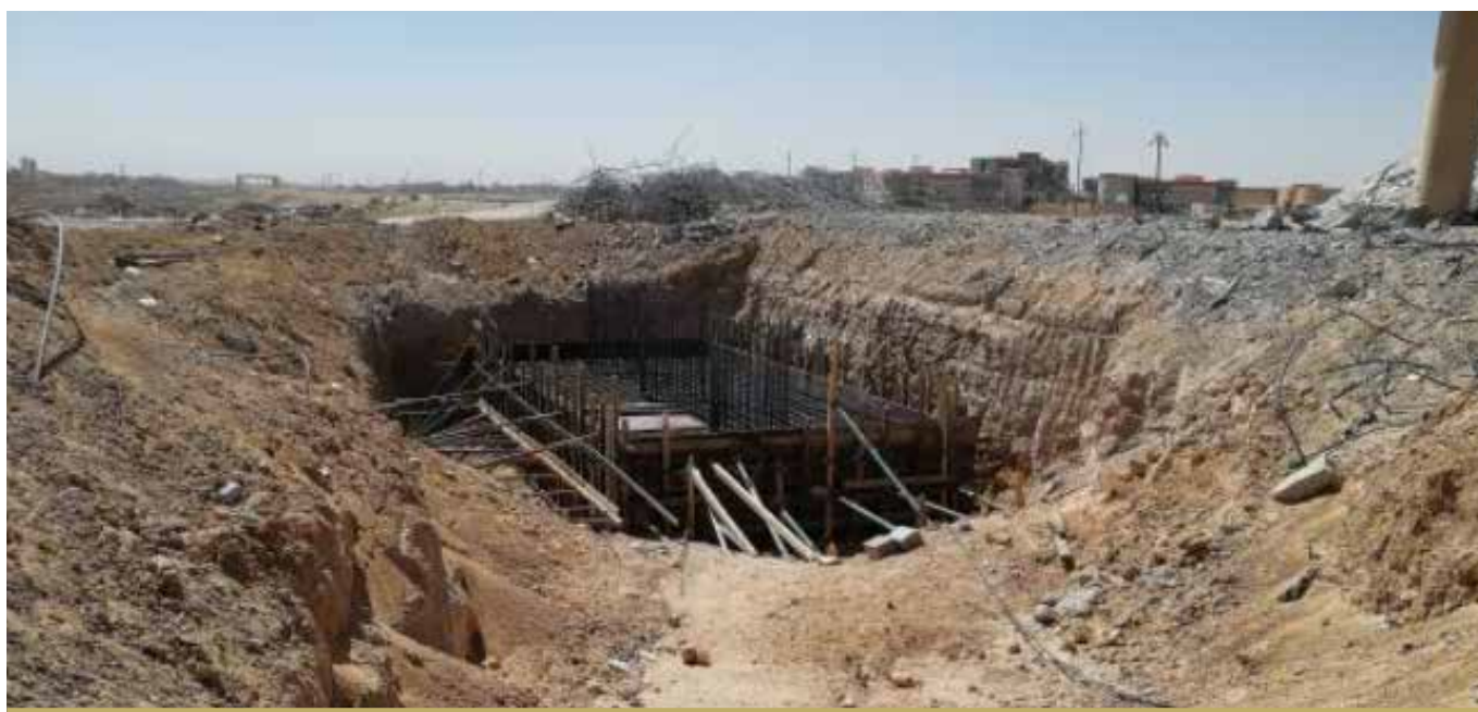
WORK WAS INITIATED ON THE UNIVERSITY BRIDGE AT ANBAR UNIVERSITY. BY THE END OF THE QUARTER, PROGRESS HAD REACHED 5%.
