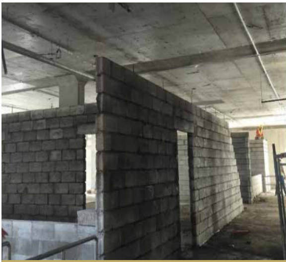
PIPES ARE INSTALLED AND BRICK WORK FOR INTERNAL WALLS AT THE TIKRIT TEACHING HOSPITAL IS ONGOING ON SITE.
