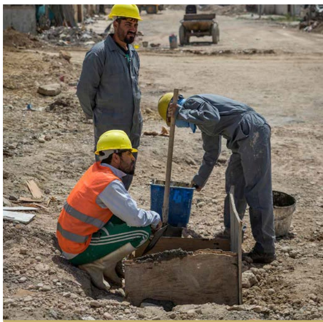
WORKERS REPAIR THE SEWERAGE SYSTEM IN THE WEST MOSUL HOSPITAL COMPLEX. THERE WERE 25 SEWERAGE PROJECTS BY THE END OF THE QUARTER IN WEST MOSUL. FFS IS COMMITTED TO PROVIDING FULL SUPPORT, WHERE FUNDING ALLOWS, FOR THE REHABILITATION OF THIS BASIC SERVICE. ©UNDP IRAQ/CLAIRE THOMAS
