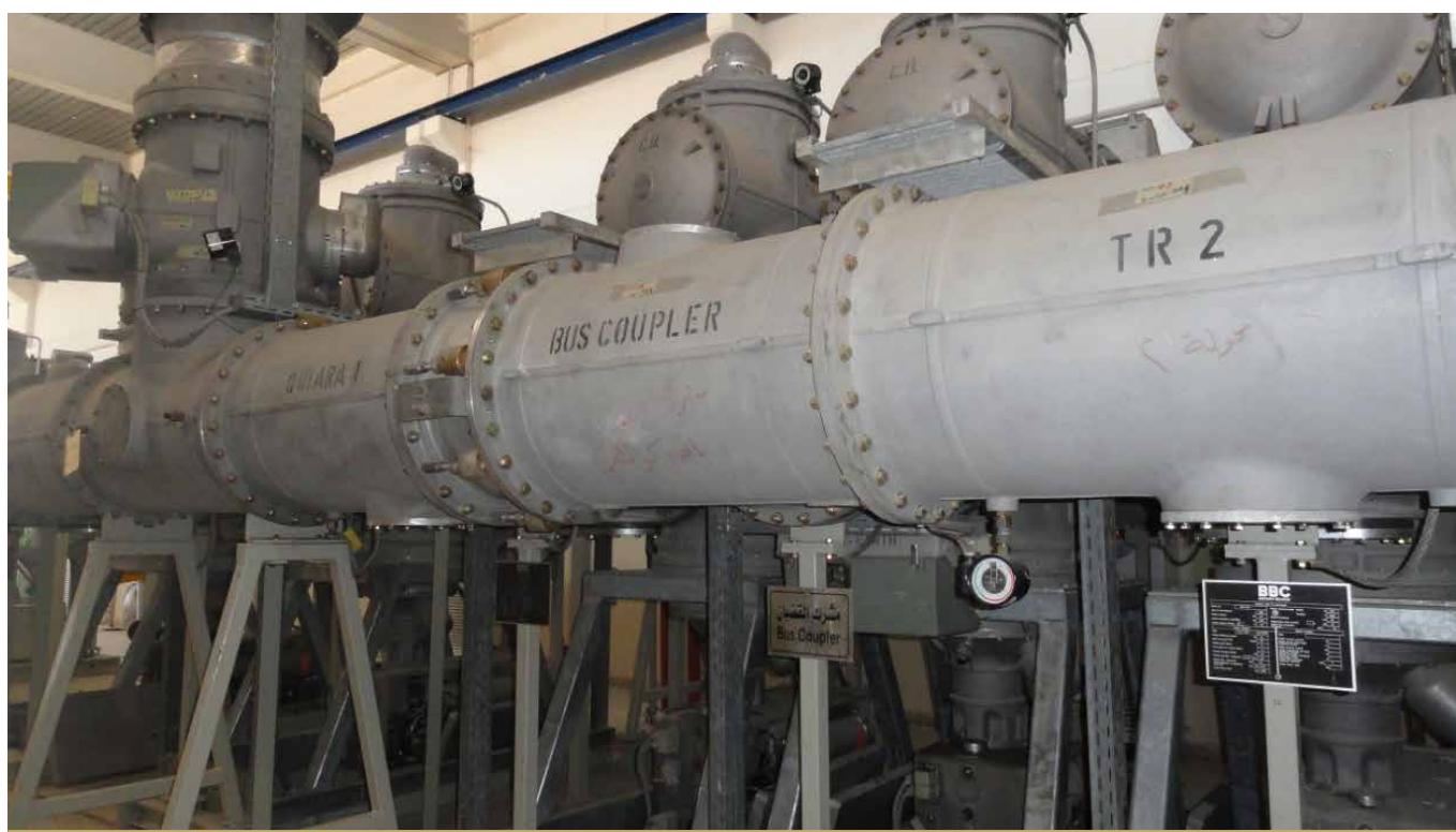
WORK ON THE SUBSTATION IN SHERGAT (PICTURED) WAS COMPLETED DURING THE REPORTING PERIOD.
