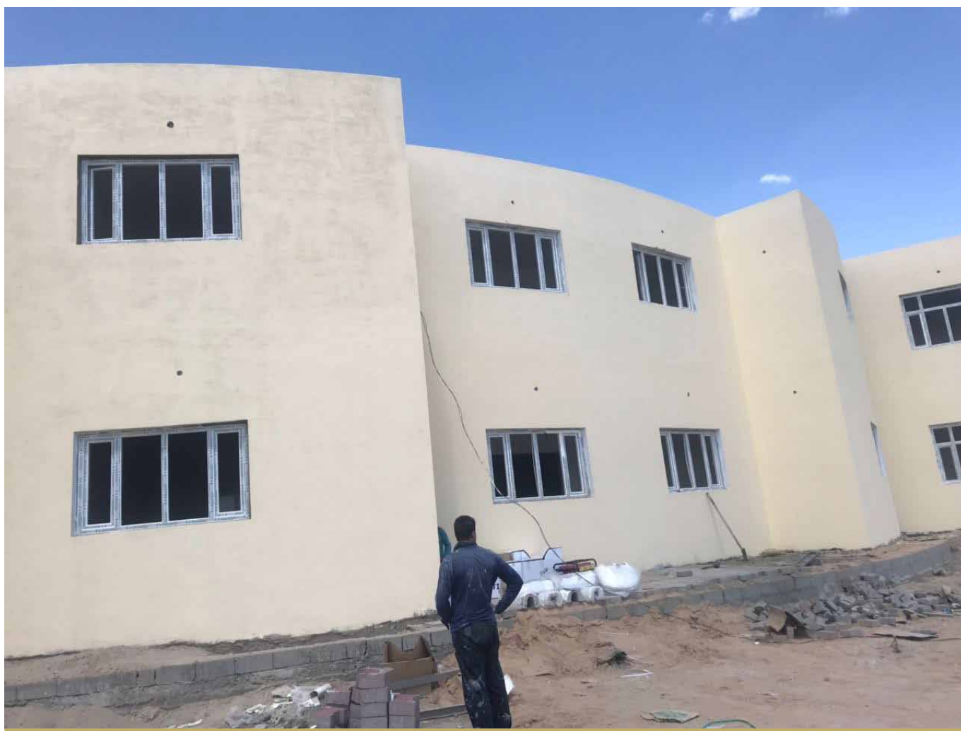
THE FALLUJAH MAYOR'S OFFICE. THE REHABILITATION OF THE OFFICE PROGRESSED SIGNIFICANTLY AND STOOD AT 95% COMPLETION BY QUARTER'S END. IT IS EXPECTED TO BE FINISHED IN THE EARLY PART OF Q3.
