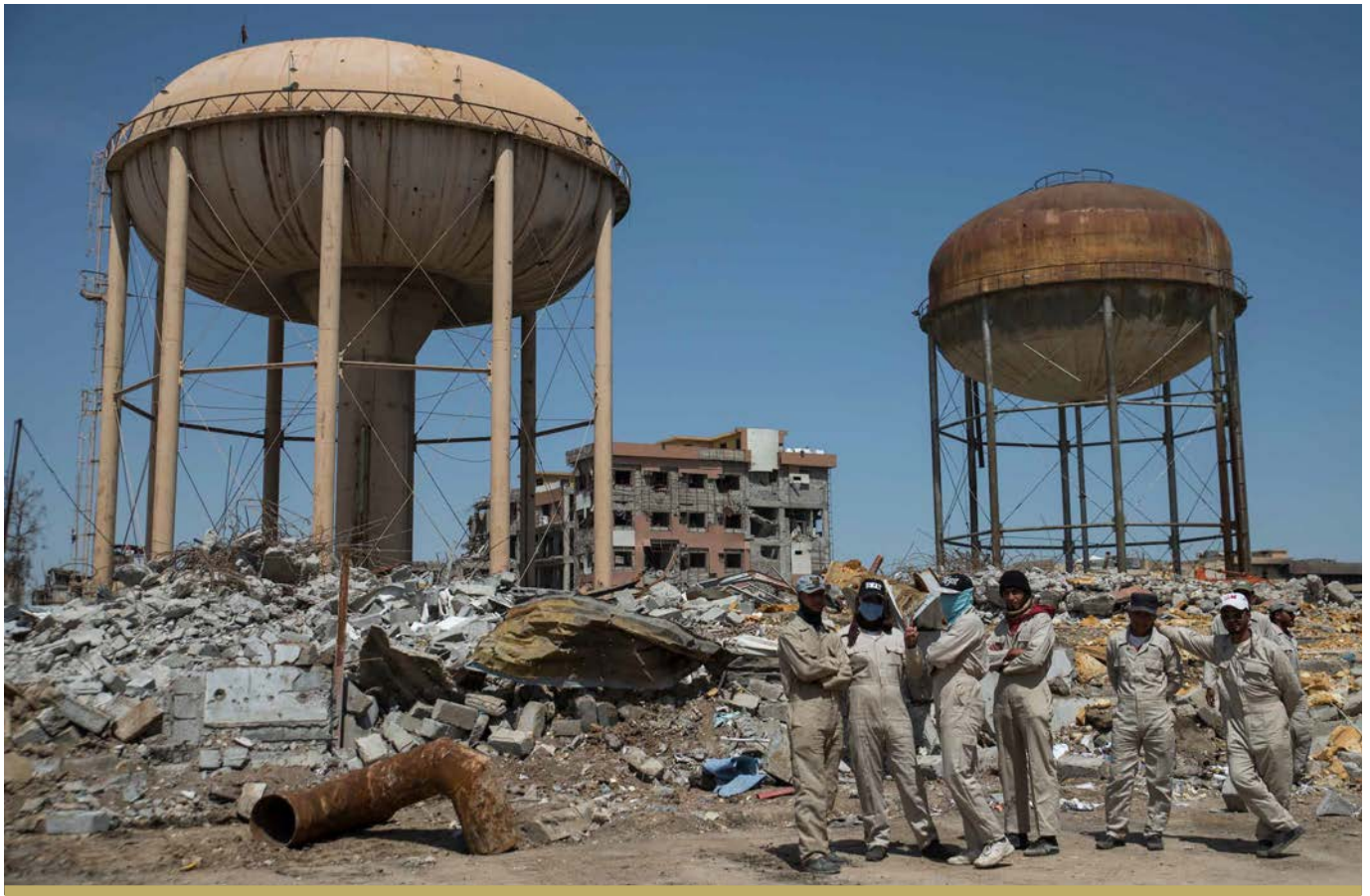
FFS SUPPORTED CASH-FOR-WORK TEAM CLEARS RUBBLE AND DEBRIS FROM AN AREA AT AL-SHIFAA HOSPITAL COMPLEX IN WEST MOSUL. ©UNDP IRAQ/CLAIRE THOMAS
