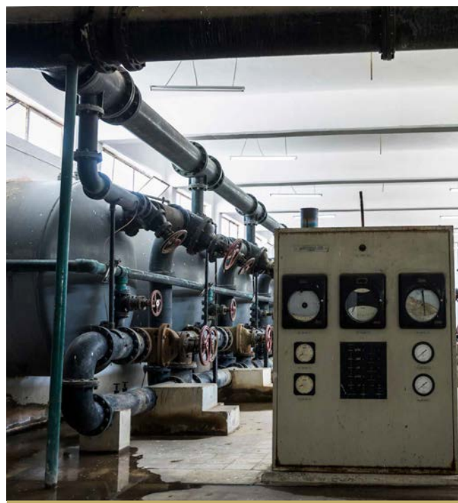
THE AL-GHIZLANI WATER TREATMENT PLANT IN WEST MOSUL. WORK PROGRESSED THROUGH THE QUARTER FROM 10% TO 45%. ©UNDP IRAQ/CLAIRE THOMAS
