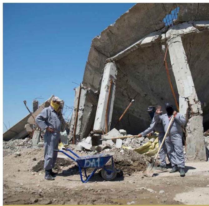
IRAQI MEN CLEAN A STREET IN THE QATHEB AL-BAN NEIGHBOURHOOD IN WEST MOSUL AS PART OF A FFS CASH FOR WORK PROJECT. BENEFICIARY FEEDBACK TO CFW PROJECT IN WEST MOSUL IS DEMANDING OVERWHELMINGLY OF THE PROJECTS, WITH BOTH LOCAL AUTHORITIES, DIRECT PARTICIPANTS, AND NEIGHBORHOODS REQUESTING ADDITIONAL SUPPORT. ©UNDP IRAQ/CLAIRE THOMAS
