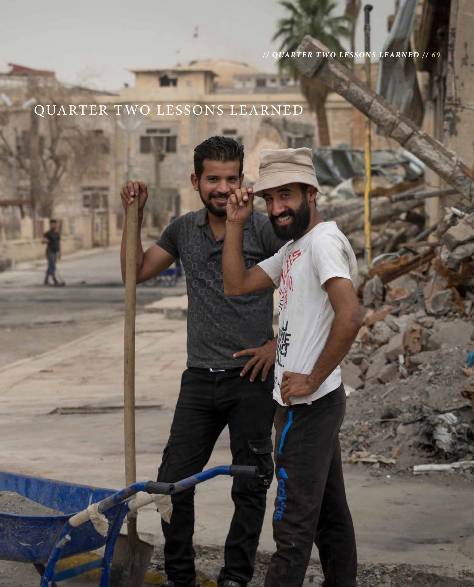
MEMBERS OF A FFS SUPPORTED CASH FOR WORK TEAM CLEAR RUBBLE AND DEBRIS FROM AN AREA AT AL-SHIFAA HOSPITAL COMPLEX IN WEST MOSUL. ©UNDP IRAQ/CLAIRE THOMAS
