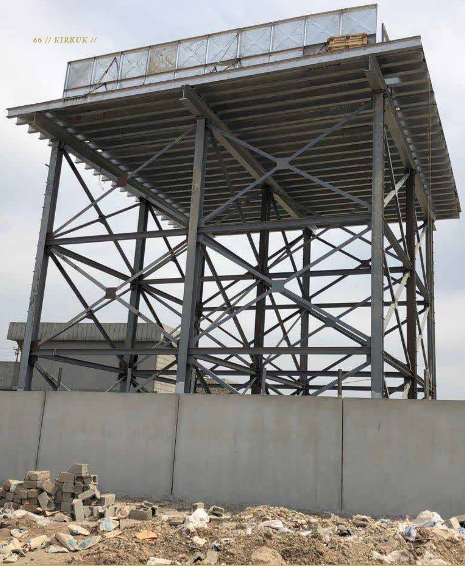
THE COMPLETED WATER TANK IN BASHIR, WHICH WAS COMPLETED IN APRIL AND NOW PROVIDES WATER FOR 350 FAMILIES.
