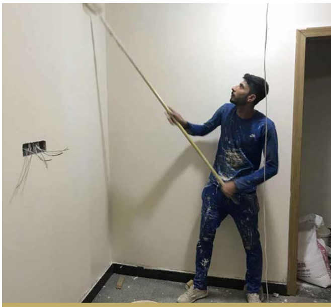
THE INSIDE OF THE FALLUJAH MAYOR'S OFFICE WHICH STOOD AT 95% COMPLETION BY QUARTER'S END. IT IS EXPECTED TO BE FINISHED IN THE EARLY PART OF Q3. FOLLOWING ITS COMPLETION, IT WILL PROVIDE A PERMANENT SUITE OF OFFICES THE MAYOR AND CITY STAFF TO SUPPORT MUNICIPAL ADMINISTRATION.
