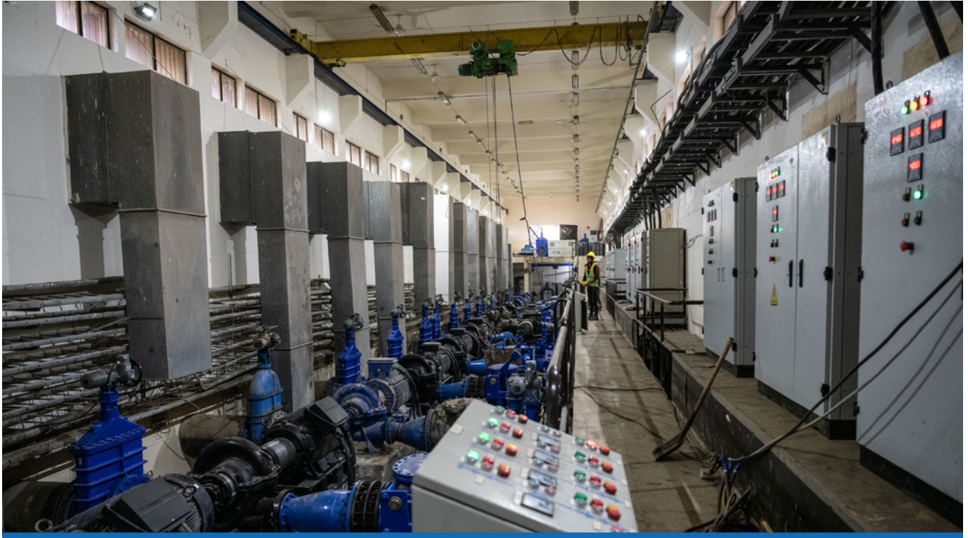
The Al Qubba Water Treatment Plant.
