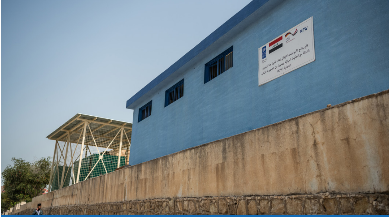
One of 21 damaged 33/11 KV substations that were rehabilitated on the Mosul University campus.
