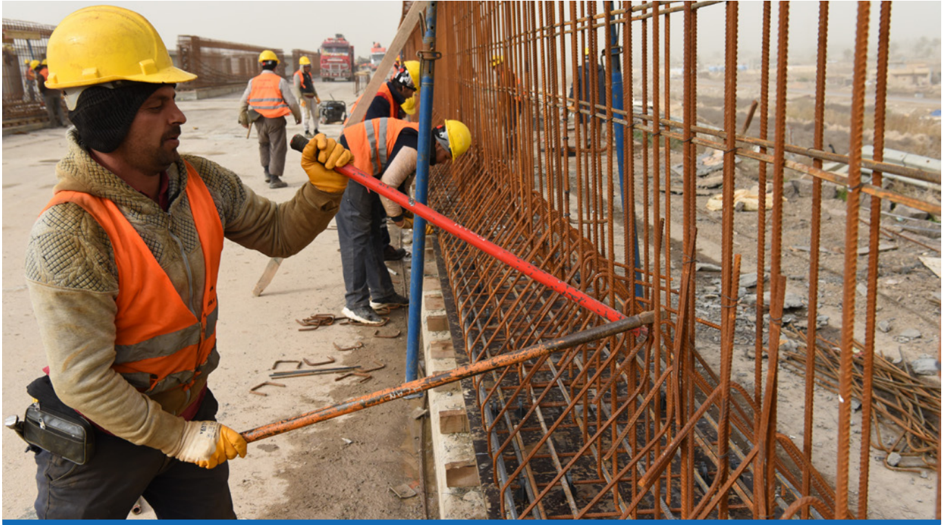
Work is ongoing at the large, two-span Palestine Concrete Bridge in Ramadi.
