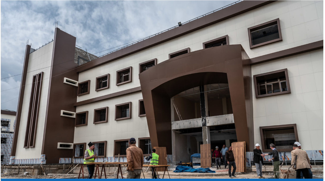
Work is underway at the Jawsach Campus of Ninewa University in West Mosul, which is being rehabilitated with the support of UNDP's FFS.
