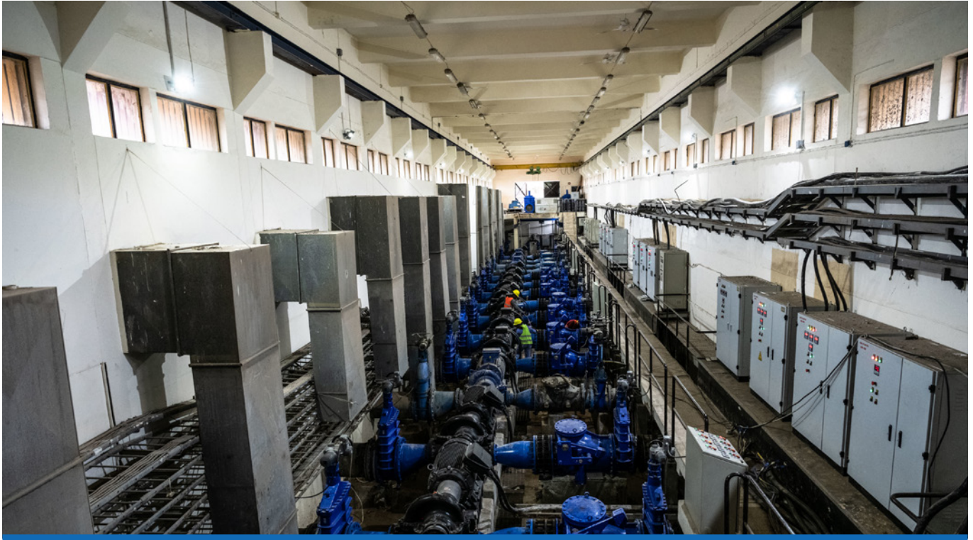
Al Qubba Water Treatment Plant, which was 80% complete at the close of the quarter.
