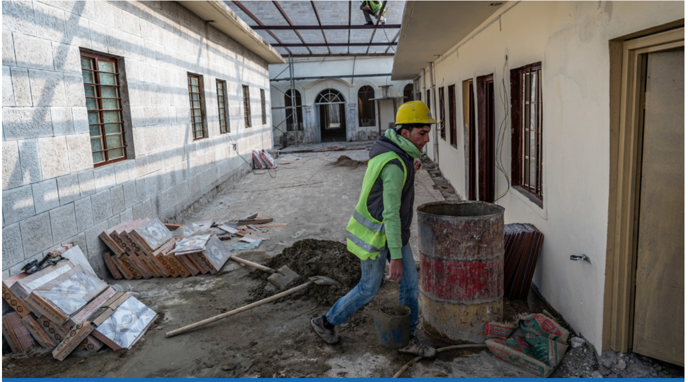
Work is underway at the West Mosul vetting centre, which was 40% complete at the end of the quarter.
