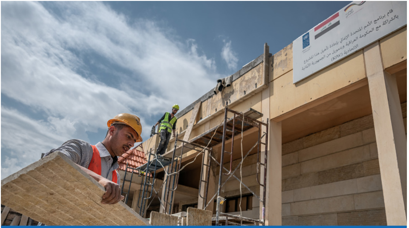
Work is underway at the Ibn Khaldoun Library at Mosul University's Second Campus.
