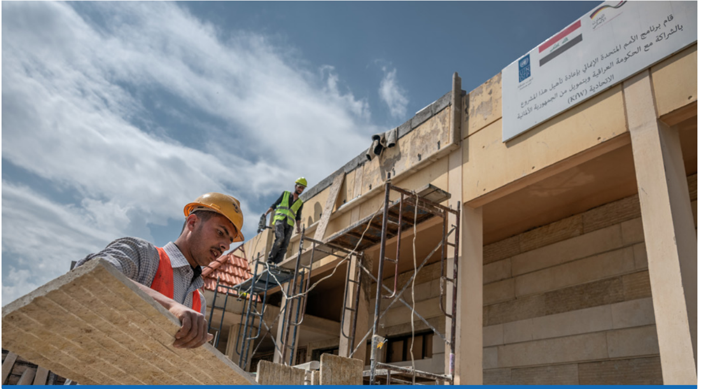
Work is ongoing to support the rehabilitation of the Baiji police station.
