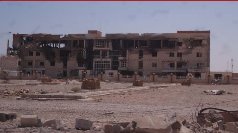
Damages to Tikrit Teaching Hospital © UN DP
