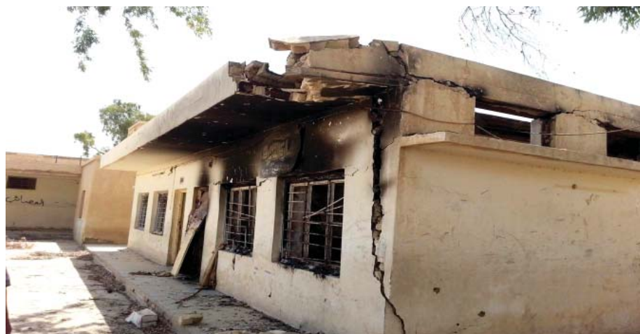
Destroyed school in Abu Ajeel, Tikrit District © UNDP
