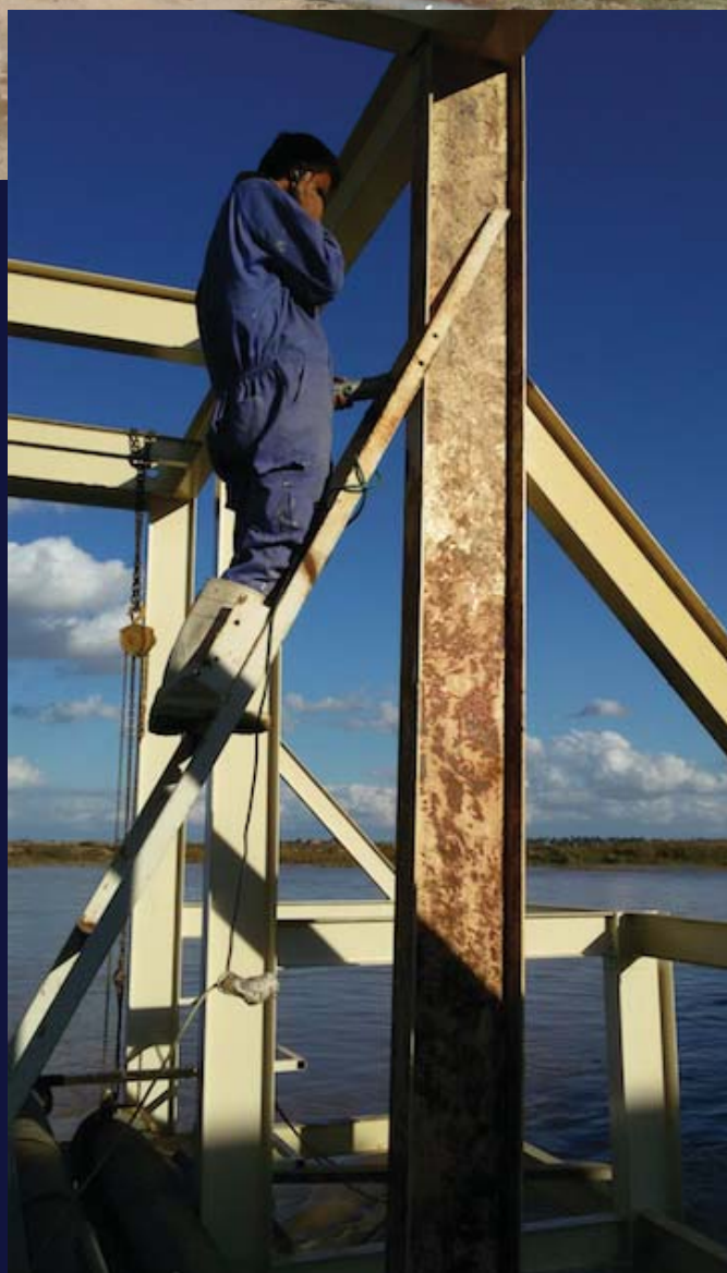
Right: Refurbishments to the Tikrit water station has supplied clean, filtered water to tens of thousands of residents. Photo credit: UNDP
