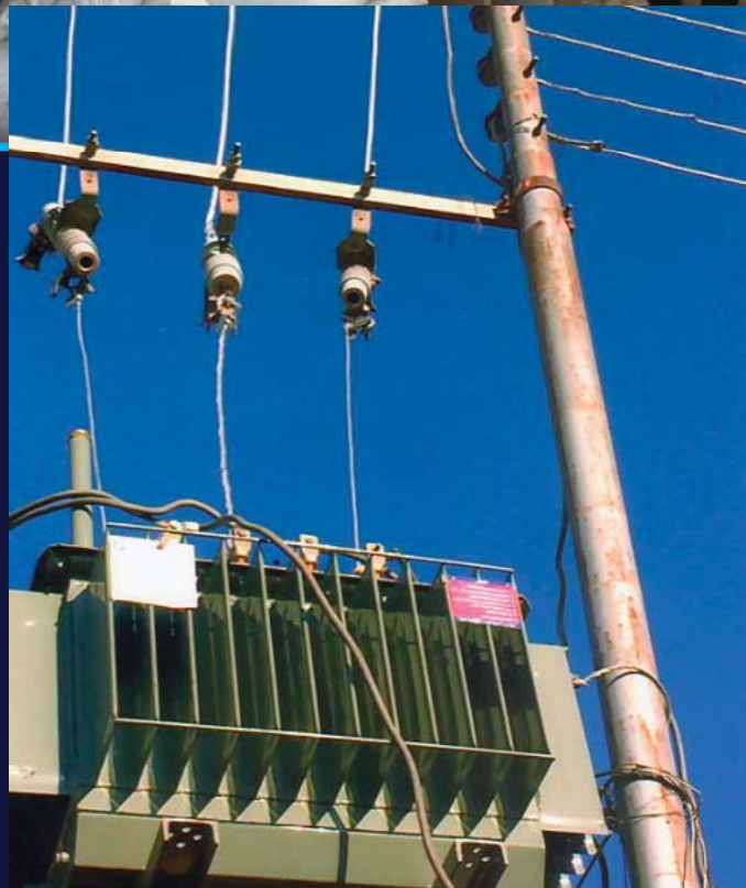
Right: FFIS supplied 50 transformers, 750 poles, and 100km of cables, which were installed by the Tikrit Electricity Department.
