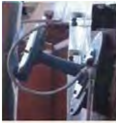
Sonic Horn Installed in Economizer.
