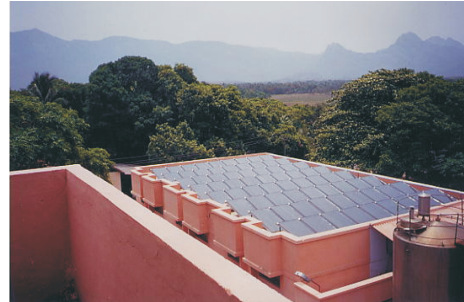
Solar Water Heating System at MILMA Dairy
