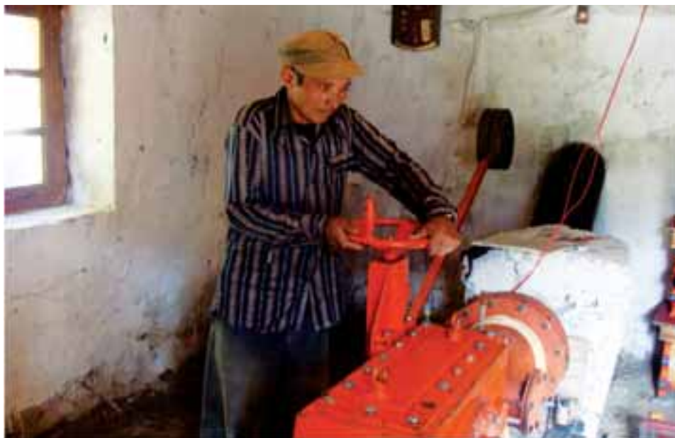
Udmaroo micro-hydro power unit
