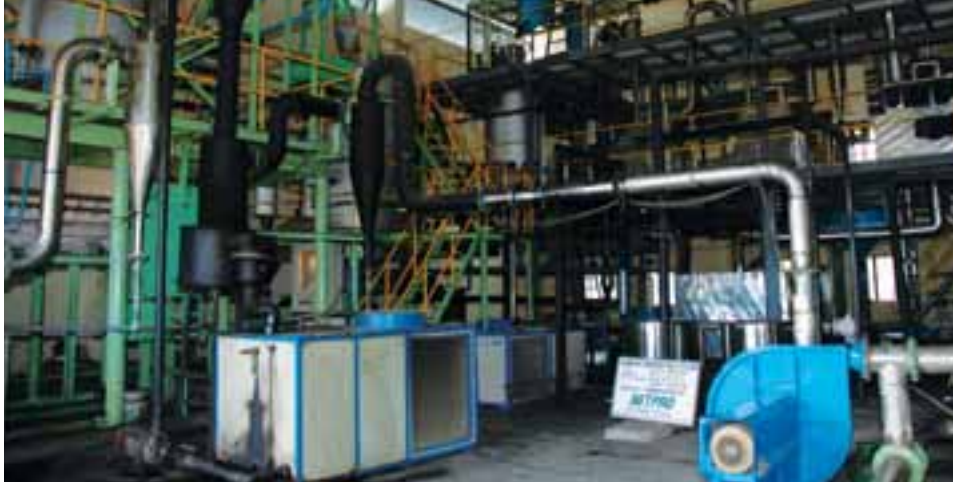
Biomass gasification system
