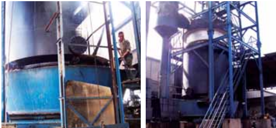
Biomass-based producer gas plant at Pulkit Steel Rolling Mills, Puducherry
