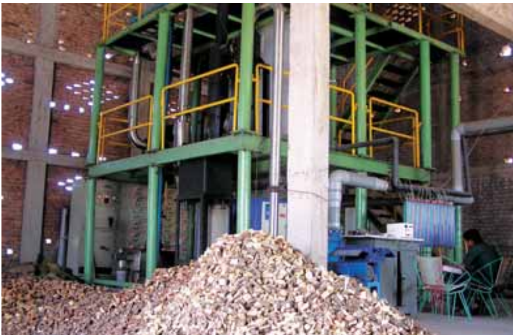
Biomass-based power plant
