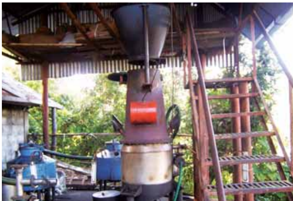
Equipment for gasification of pine needles
