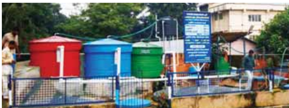
Biogas unit in Pathanapuram
