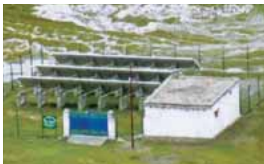
Solar photovoltaic power plant at Juldo
