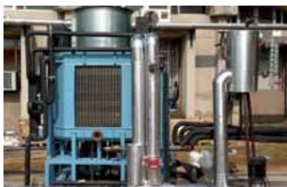
Parabolic Troughs coupled with Air Cooled Double-effect Vapour Absorption Machine (15 kW Cooling Capacity)
