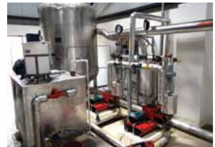
Vapour Absorption Machine being used for cooling
