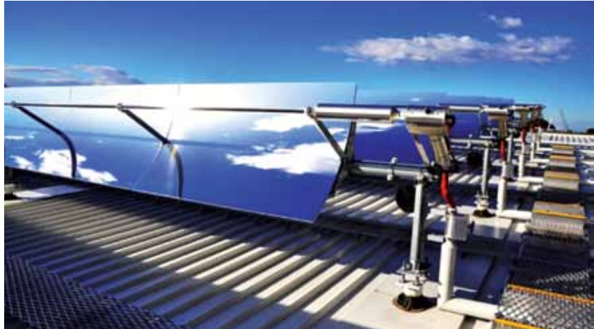
Solar Cooling System at Charlestown Square, Australia
