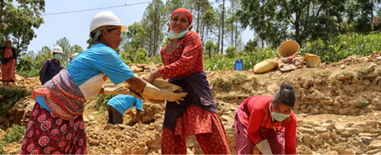
Women engaged in the rebuilding effort, in Sindhupalchok district, under UNDP's cash for work programme.
