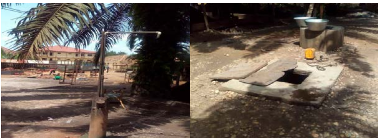
Standpipe (left) and well (right)
