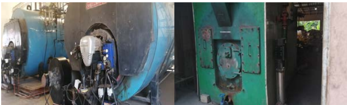
Steam boilers encountered in industries
