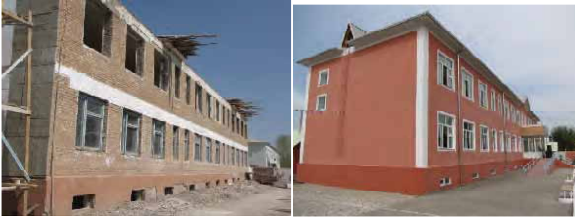
Renovation of school, Fergana region. Measures implemented by the EEPB project resulted in heat energy savings of 60 percent.
