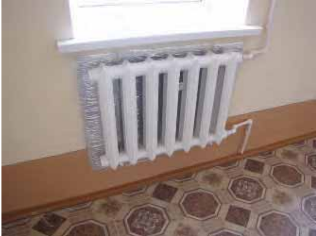
Reflective insulating panel behind radiator
