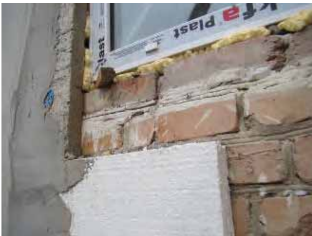
Wall insulation, window sealing, and plastic frames with sealed glass
