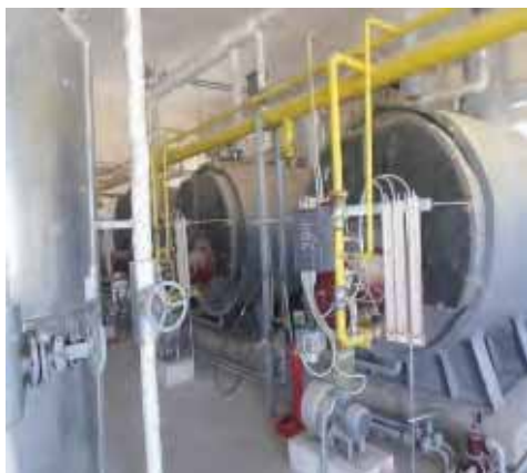
High-efficiency boilers, Urgench airport
