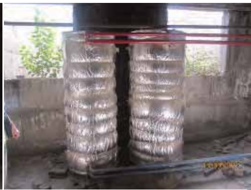
Insulation at heat exchanger at district heat entry point of forensic building, Tashkent
