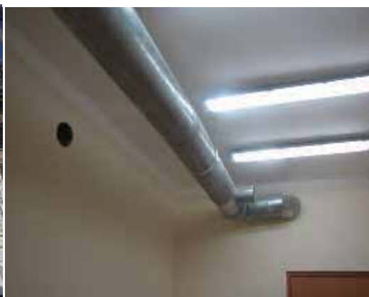
Air duct in Tuzel clinic
