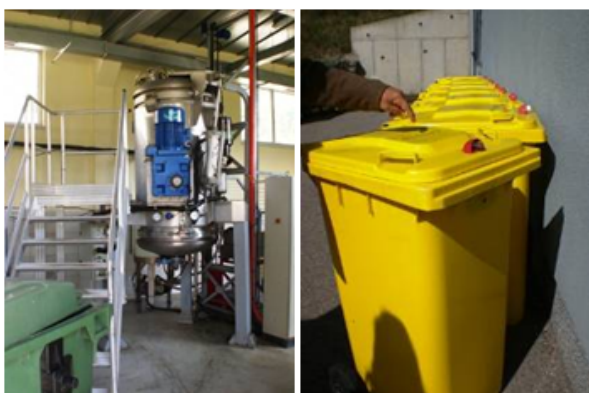
Bio-hazardous waste treatment facility at General Hospital Doboj: Steam treatment system (left), collection and transport container for infectious waste (right)
