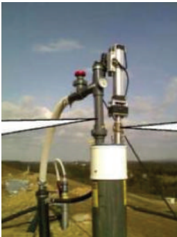
Figure 16 (left). Ground LFG collection equipment. A pipe for filtrate collection (right), a pipe for LFG collection (left)
