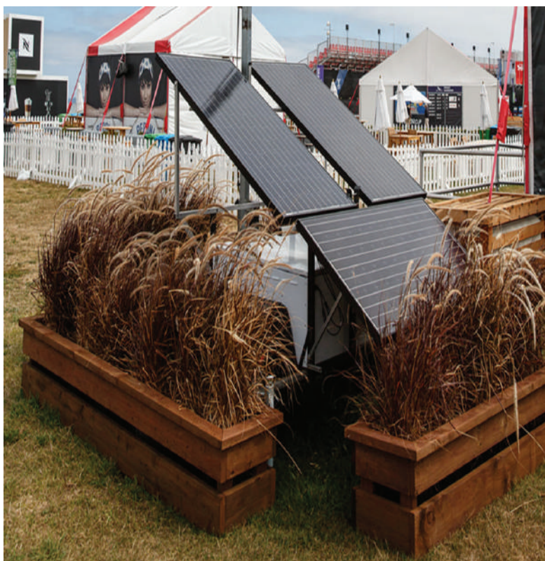
Figure 12. Small scale temporary solar PV providing cost-effective off-grid lighting at the 34th America's Cup (Source: Anthesis Consulting Group)
