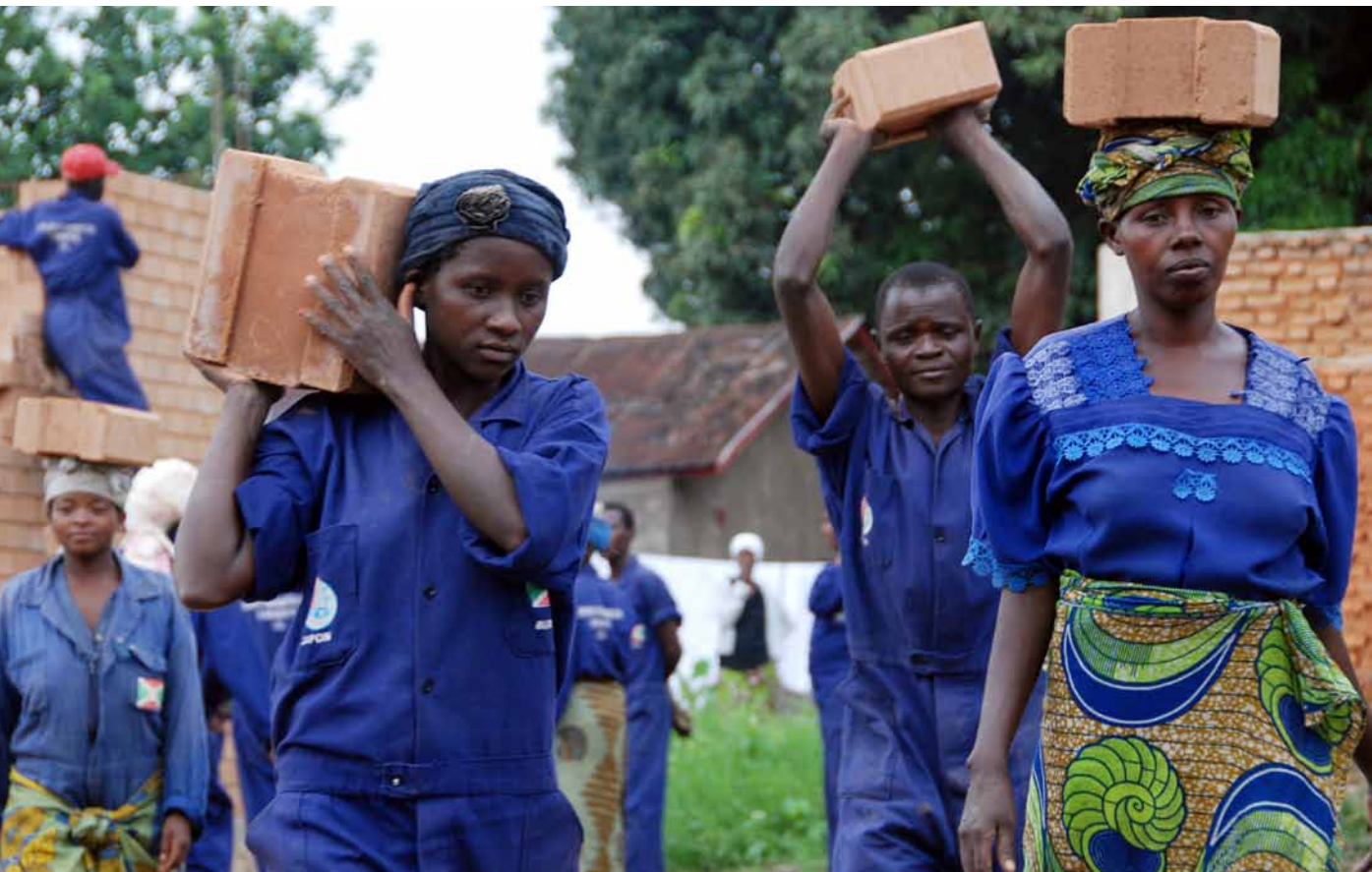
Livelihoods and economic social recovery project in Burundi. Micheline Bazima, a mother of 7 working on the Buruhukiro Road rehabilitation project in Nyagasaka village, Burundi. ©UNDP Burundi
