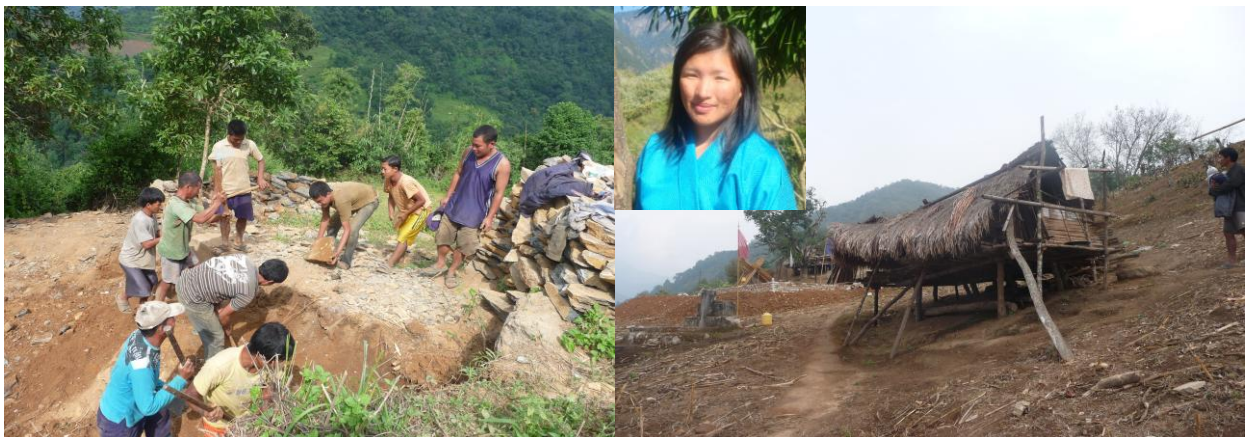
Figure 32: Community labour contribution in building new houses (left). Tashi Tsomo (inset), a student in Sonamthang High School, said that her birth place of Lamtang is in the process of reincarnating into a new Lamtang.
