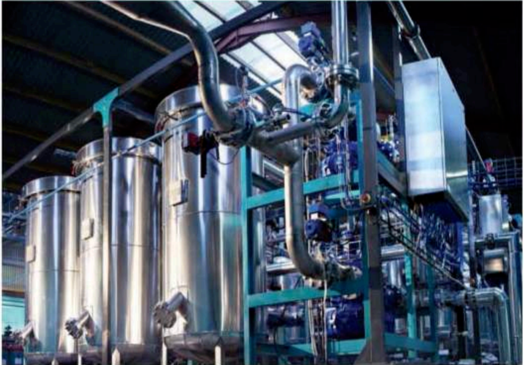
Figure 30: Liquefied Biogas facility - Source (GTS)
