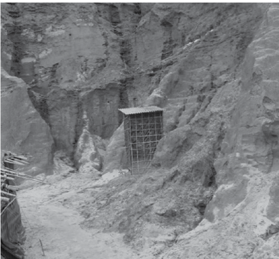
Latrine under the eroded hill slope | Photo: UNDP Bangladesh/Arif Faisal
