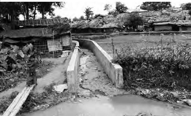
Surface water drainage in the camp | Photo: UNDP Bangladesh/Arif Faisal
