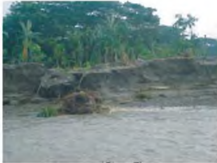
Riverbank erosion at Kutuba, Bhola
