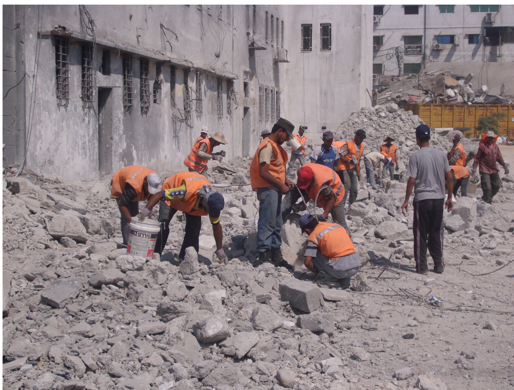
UNDP/PAPP and its partners ensured that sorting of debris was performed on-site through labour-intensive methods before it was sent on to crushing or dumping sites, which gave local home owners the opportunity to reclaim personal belongings and recyclable materials. Of 480,000 tons of debris removed through the project, the majority was crushed and eventually reused in road rehabilitation initiatives by UNDP, NGOs, and local institutions. Photo credit: UNDP PAPP
