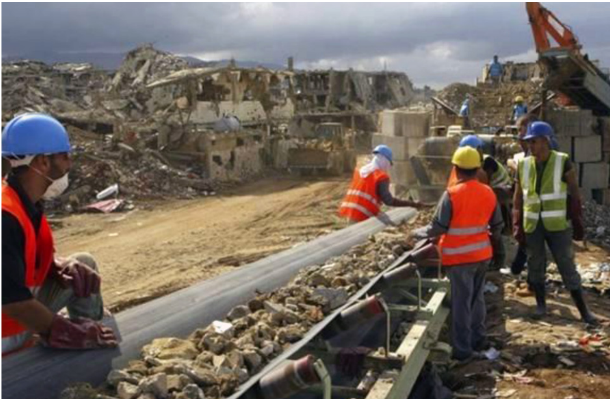
UNDP's multiple debris management initiatives in Lebanon have all centered on the principle of community ownership and engagement. As part of the Nahr-El-Bared Camp (NBC) project, shown here, community members shown are engaged in the process of sorting and crushing some 500,000 cubic meters of debris, for further treatment and reuse. Photo credit: UNDP Lebanon.
