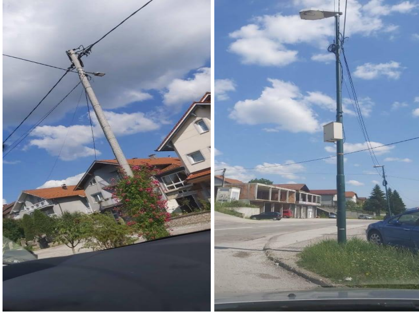
Image 26: Poles (Reinforced concrete - left, metal – desno)
