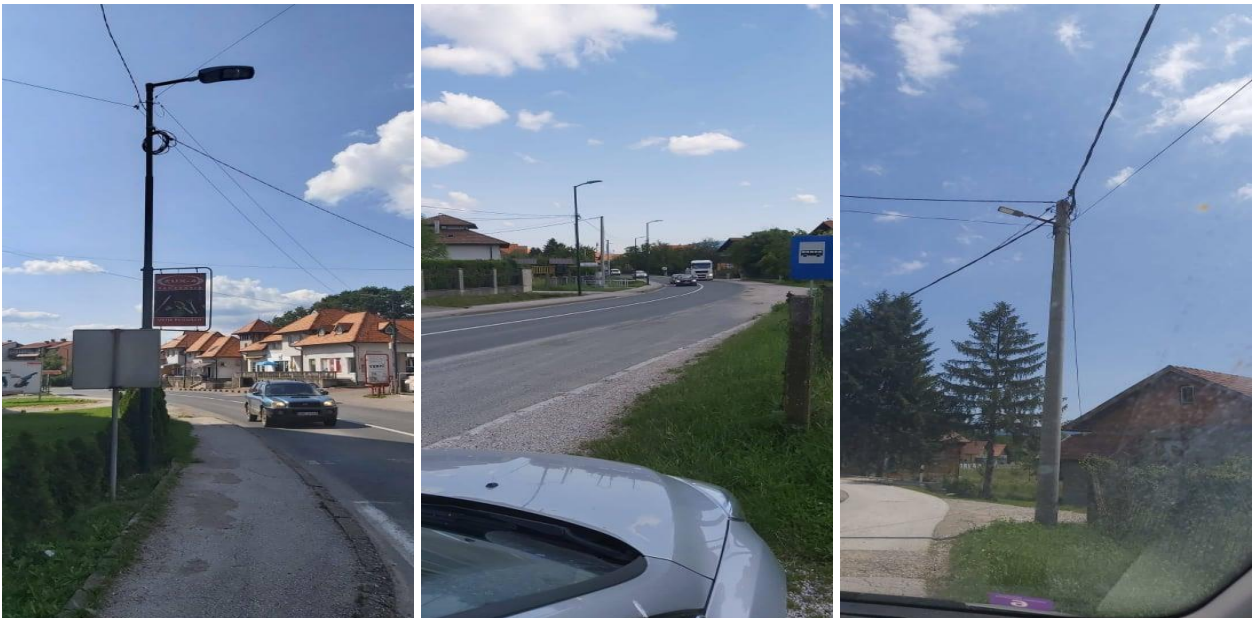
Image 28: Poles (unauthorized cabling - left, under ground cabling – centre, over ground cabling – right)
