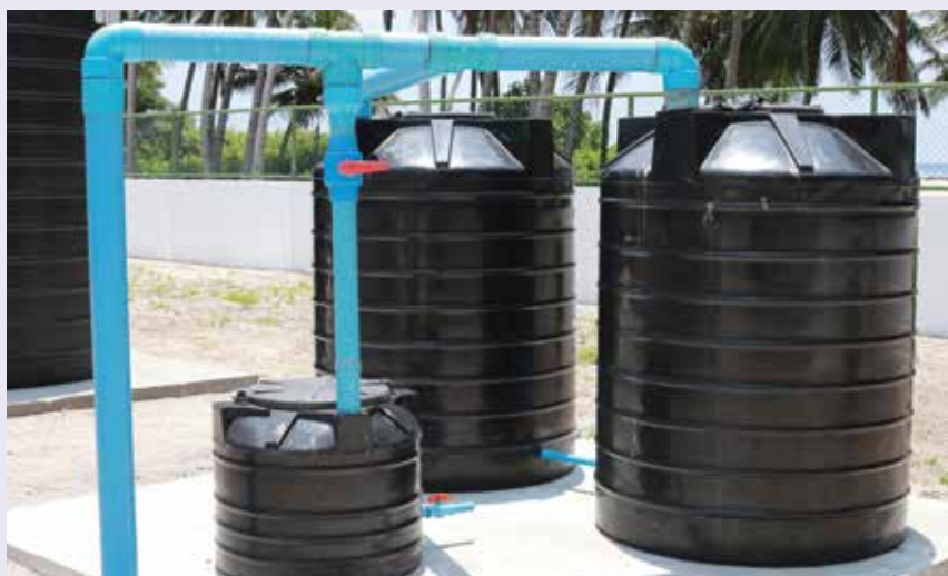
▲ Water collection system in an island. © UNDP Maldives
