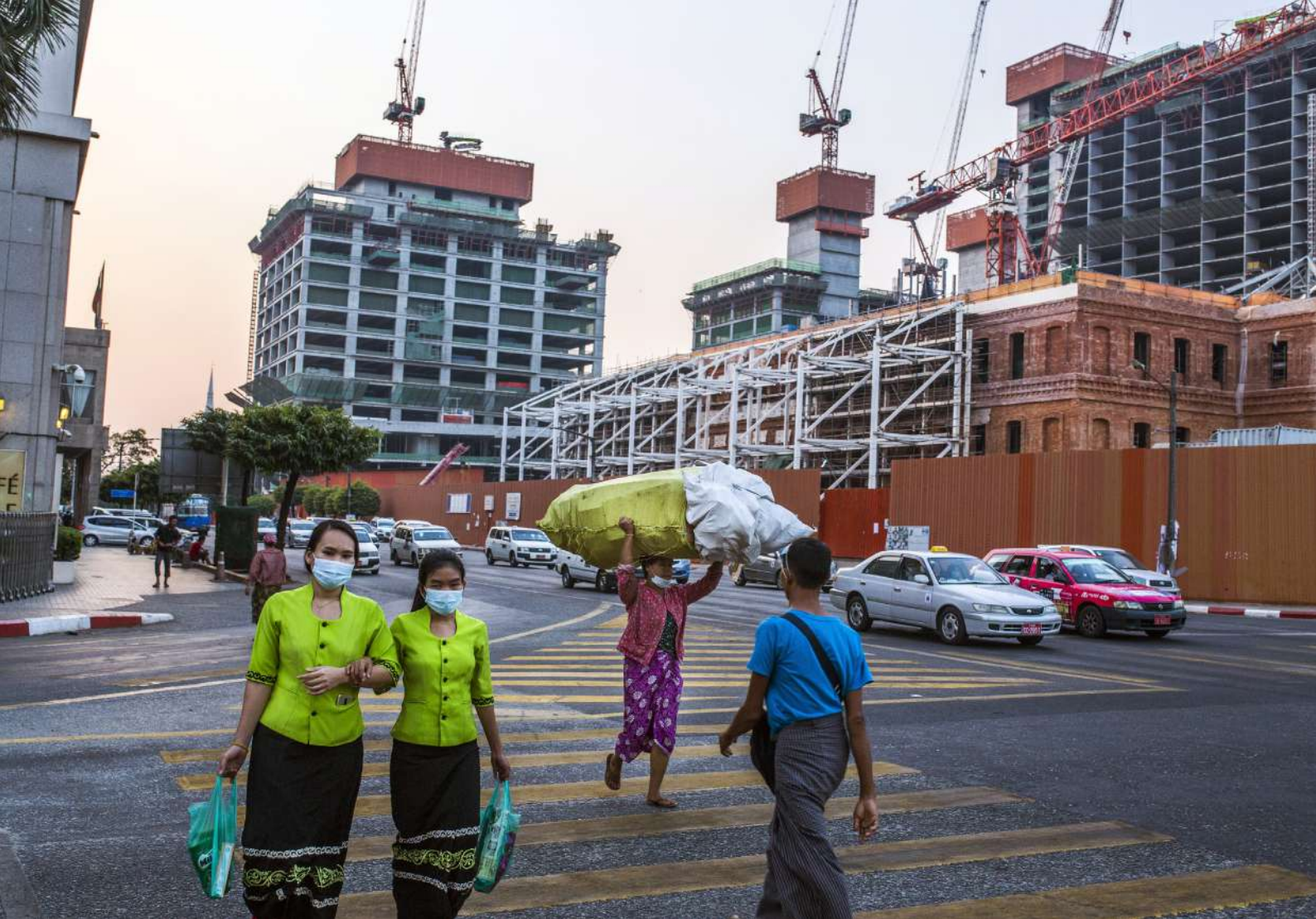
February 2021: People pass by the construction site, where work is suspended, of what was to become one of the largest hotel and shopping mall complexes in Yangon. ©M.O
