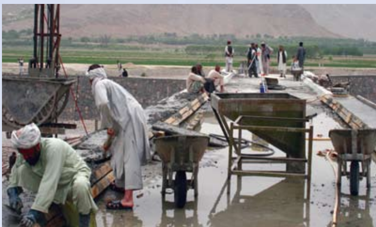
As part of National Area Based Development Programme Arghandab Bridge under construction in Kandahar
