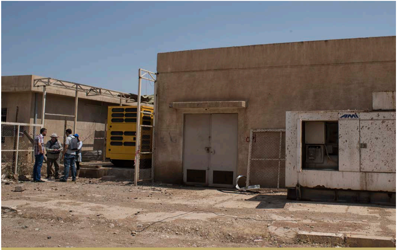
A NEW GENERATOR (LEFT) AT MOSUL UNIVERSITY REPLACES A DAMAGED GENERATOR (RIGHT) . EIGHT GENERATORS HAVE ALREADY BEEN DELIVERED, HELPING SUPPLY THE INSTITUTION WITH ELECTRICITY WHILE STUDENTS COMPLETE EXAMS. © UNDP IRAQ / MACKENZIE
