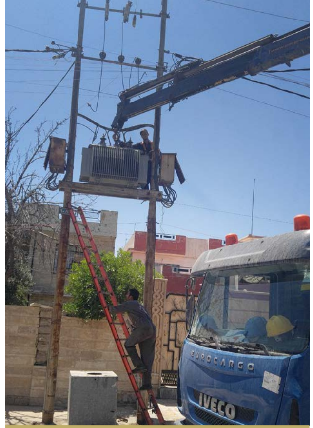
DISTRIBUTION TRANSFORMERS ARE INSTALLED TO SUPPORT THE RESTORATION OF THE ELECTRICITY NETWORK IN EAST MOSUL. © UNDP IRAQ / ABDULLAH SABER
