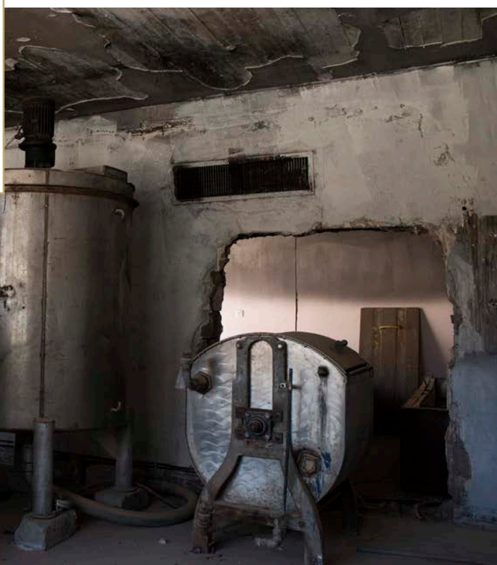
A ROOM IN A WOMEN'S DORMITORY AT MOSUL UNIVERSITY WAS USED BY ISIL TO PRODUCE EXPLOSIVES AND NEEDS EXTENSIVE REPAIRS. © UNDP IRAQ / LINDSAY MACKENZIE
