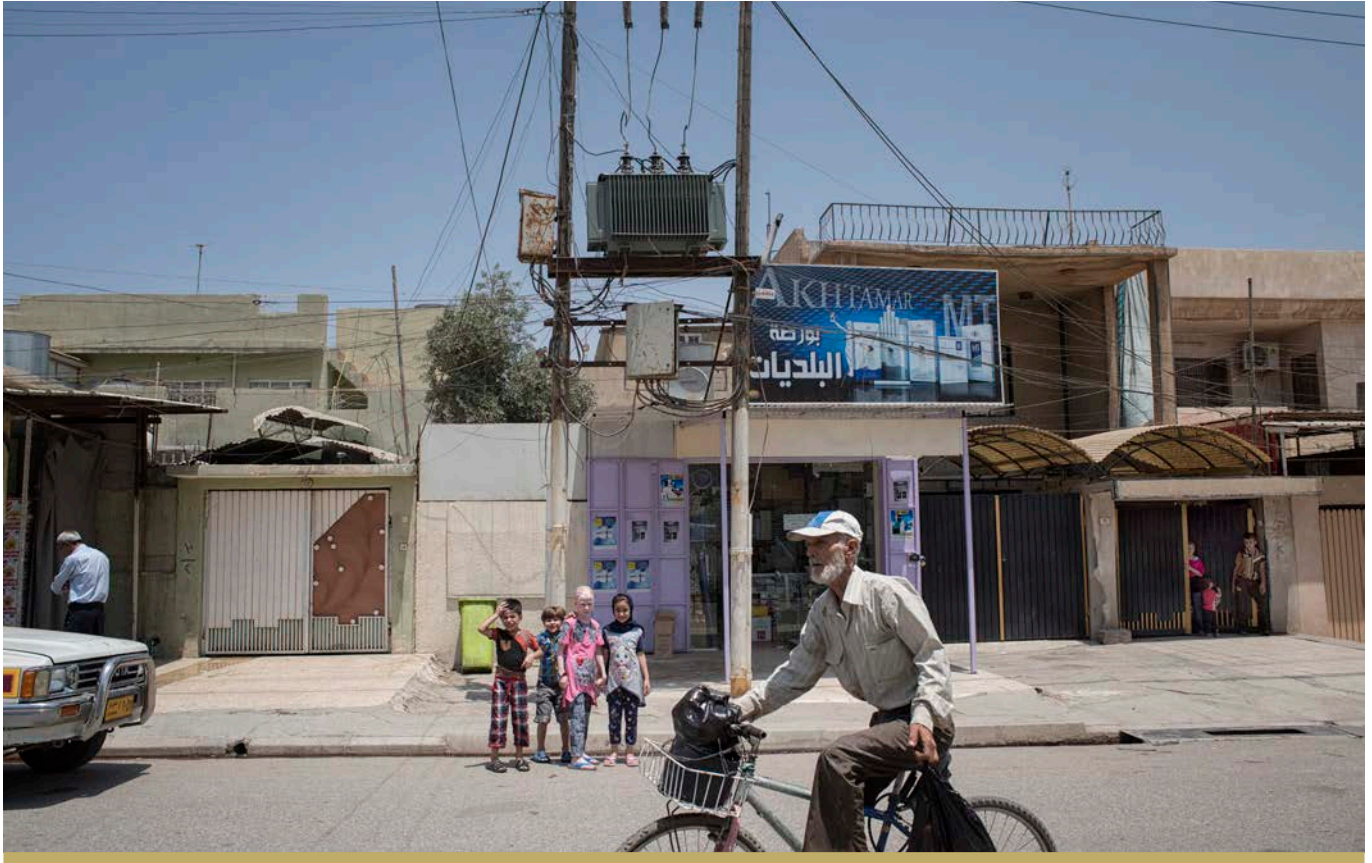
CHILDREN STAND BELOW A NEW DISTRIBUTION TRANSFORMER - ONE OF 270 INSTALLED IN EAST MOSUL. © UNDP IRAQ / MACKENZIE
