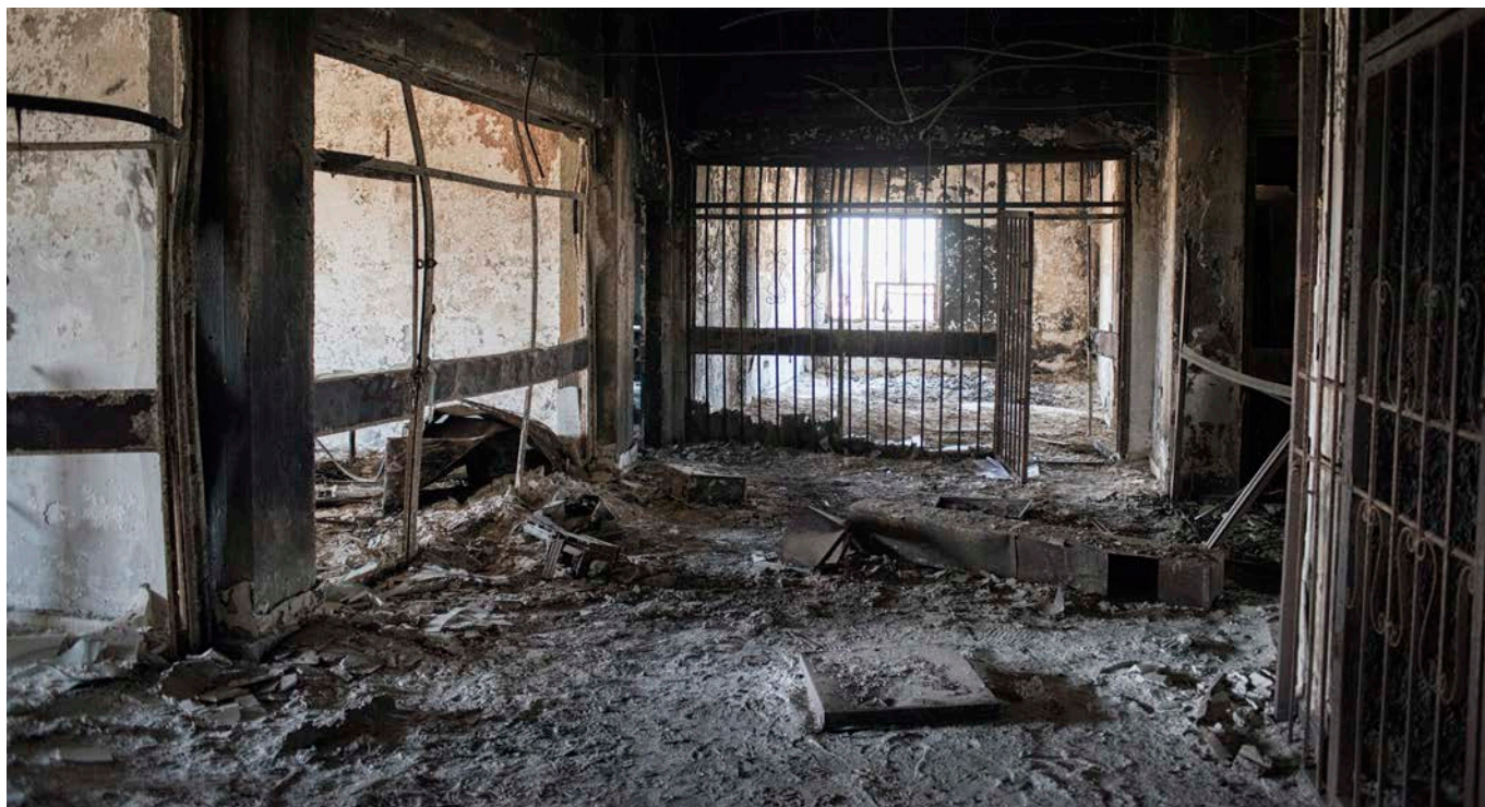
DAMAGED ADMINISTRATIVE OFFICES IN WEST MOSUL GENERAL HOSPITAL. © UNDP IRAQ / LINDSAY MACKENZIE
