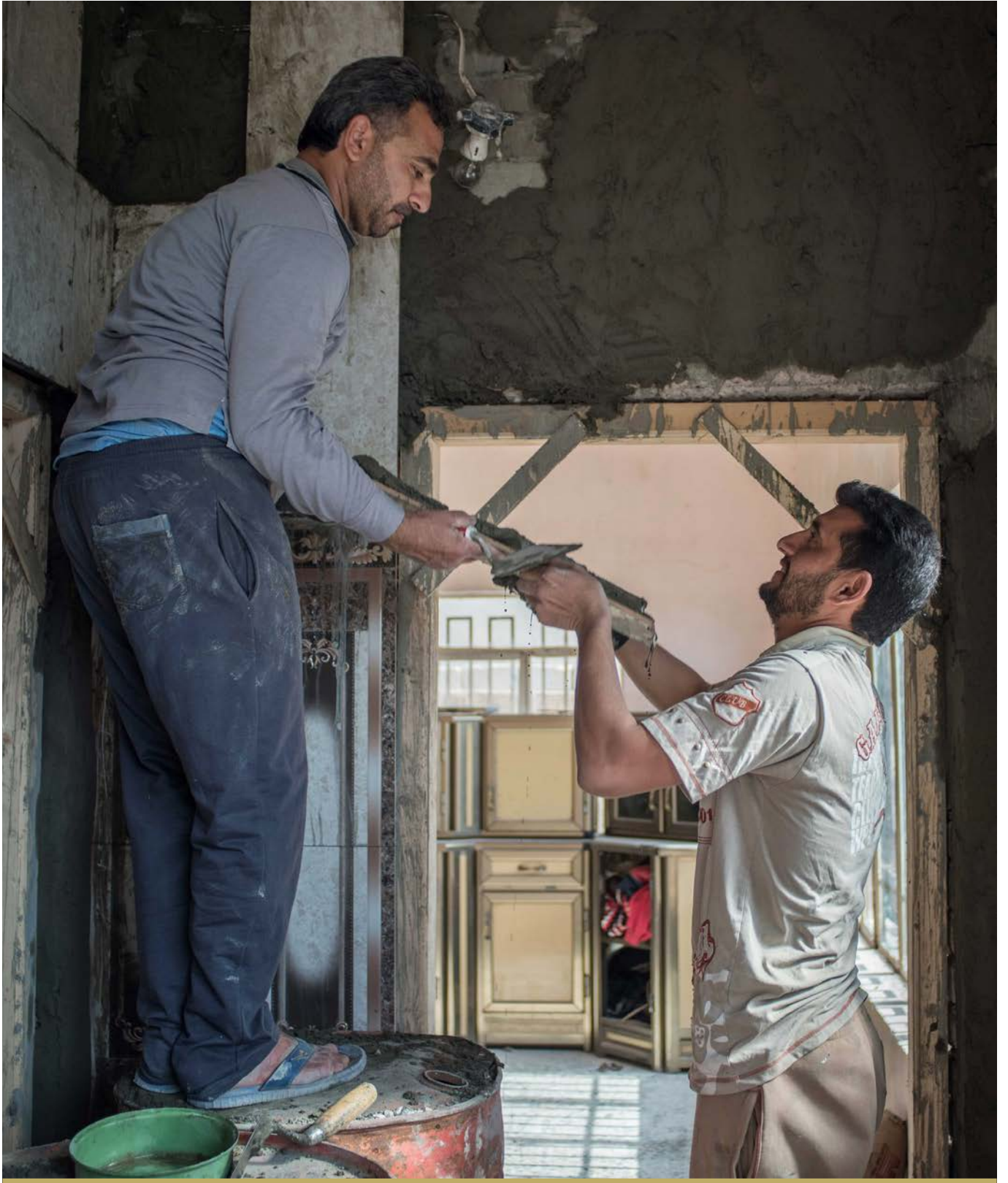
NEIGHBOURS WORK TOGETHER TO REPAIR A HOME IN FALLUJAH. © UNDP IRAQ / LINDSAY MACKENZIE
