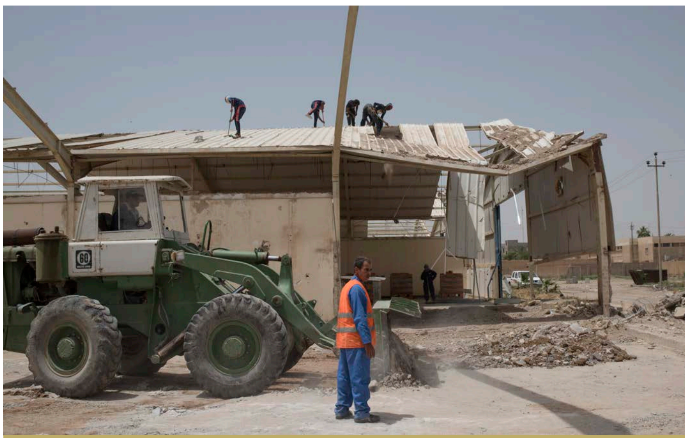
WORK CONTINUES ON THE VOCATIONAL TRAINING CENTER IN RAMADI. © UNDP IRAQ / LINDSAY MACKENZIE
