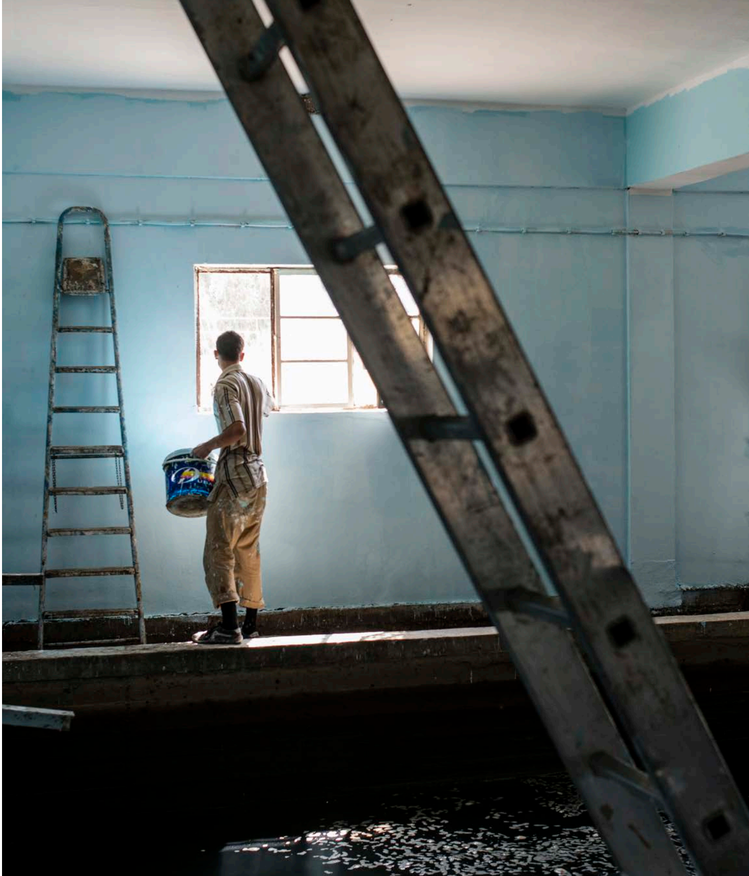
WORKERS PAINT THE WALLS AROUND NEWLY-REPAIRED FILTERING TANKS IN EAST MOSUL'S AL QUSOR WATER TREATMENT PLANT. THE PLANT IS ALREADY PROVIDING SAFE WATER TO MORE THAN 300,000 PEOPLE. © UNDP IRAQ / ALEX POTTER
