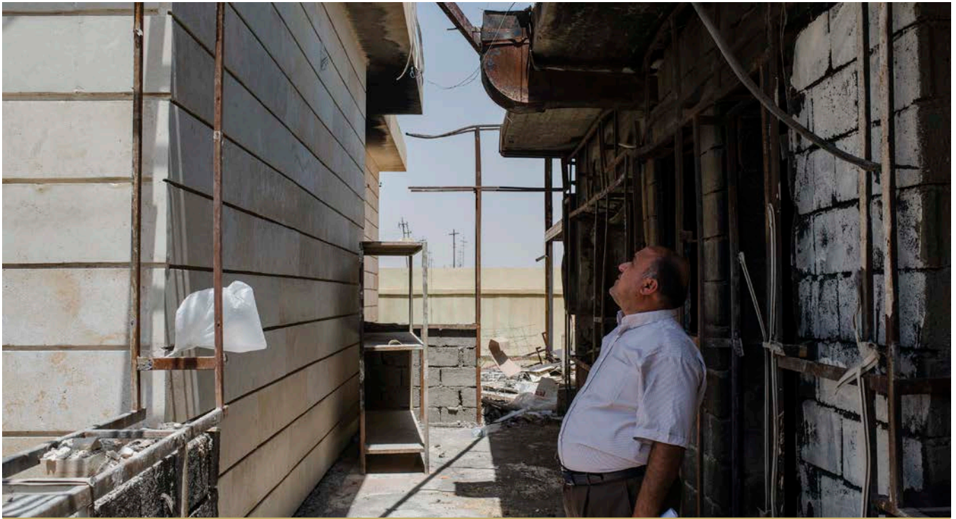
AN ENGINEER COMPARES A BUILDING AFTER REHABILITATION (LEFT) WITH ONE YET TO BE REPAIRED AT HAMDANIYA HOSPITAL. THE NEW LIMESTONE COVERING FOR THE NEW BUILDING WAS SOURCED LOCALLY. © UNDP IRAQ / ALEX POTTER
