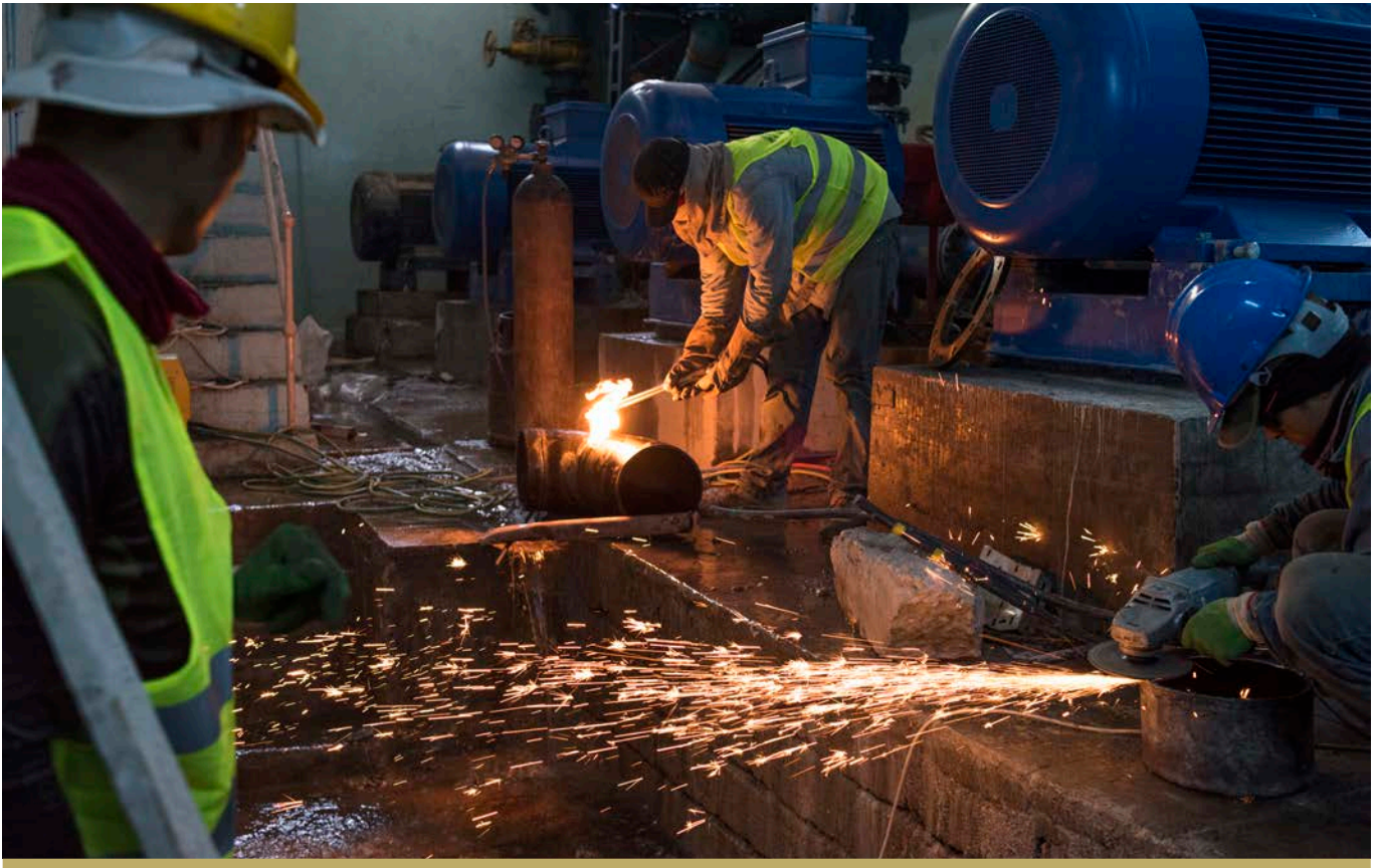
WORK AT AL QUSOR WATER TREATMENT PLANT, WHERE REHABILITATION IS 85 PERCENT COMPLETE. © UNDP IRAQ / LINDSAY MACKENZIE
