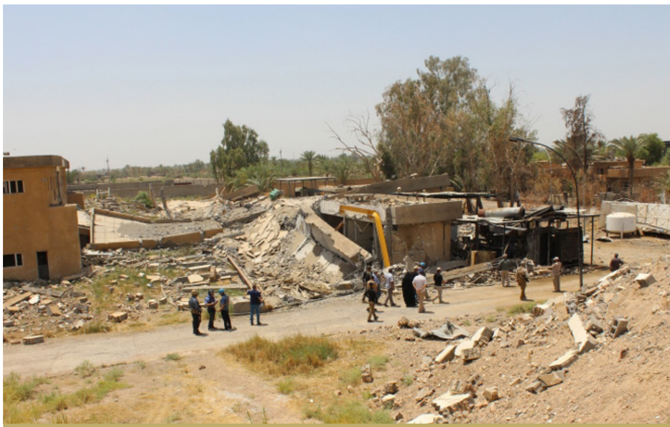
AL AZRAKIYAH WATER TREATMENT PLANT BEFORE REHABILITATION IN AUGUST 2016. © UNDP IRAQ
