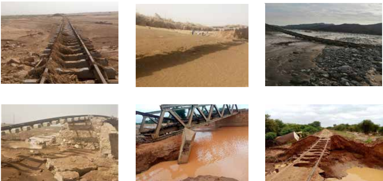
FIGURE 10 - 7: Selection of photos showing the extent of the National Road damages due to the 2020 floods
