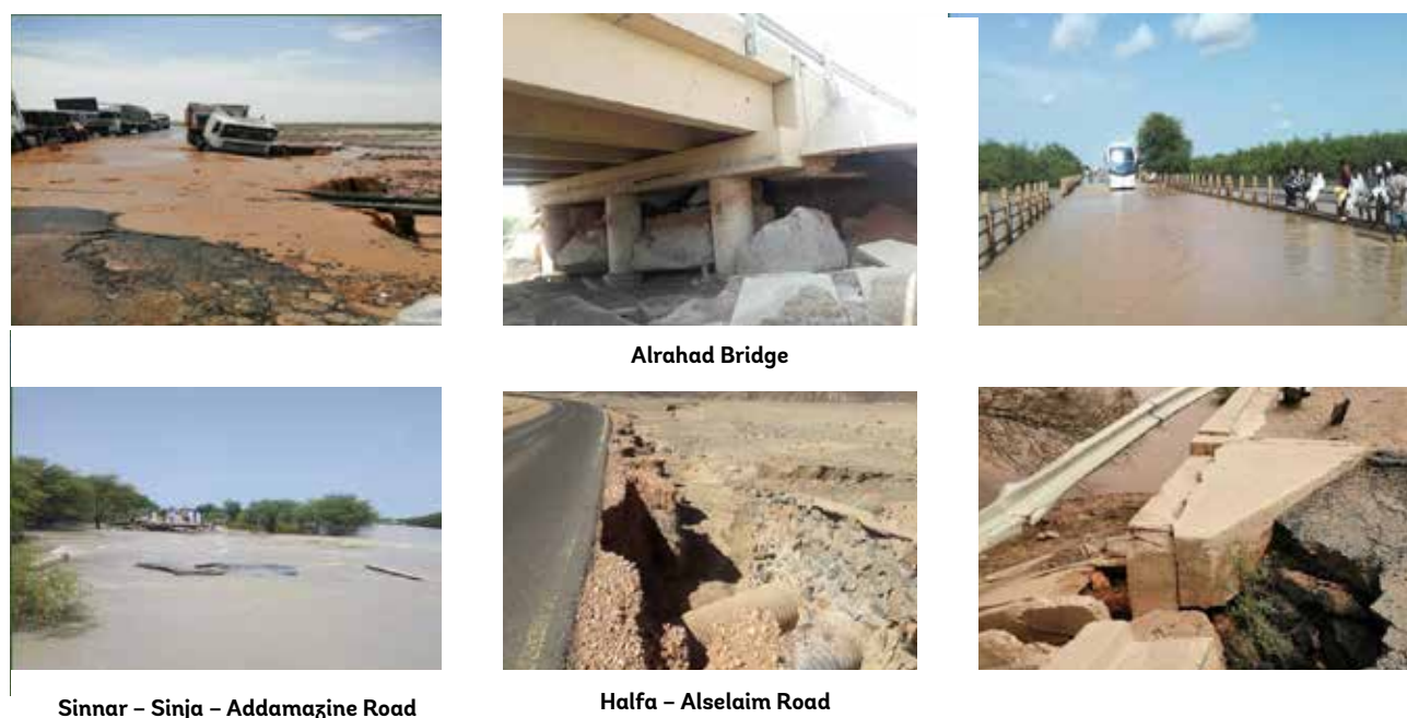
FIGURE 10 - 6: Selection of photos showing the extent of the National Road damages due to the 2020 floods
