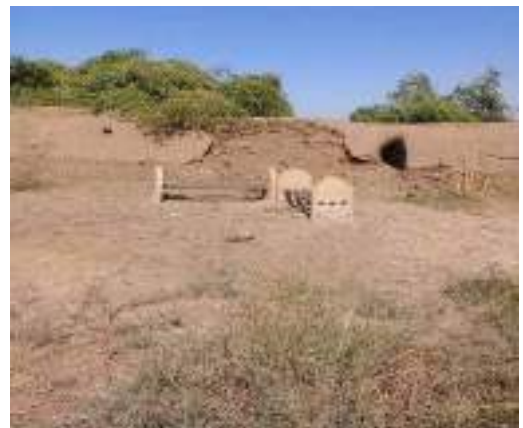
FIGURE 15 - 2: Partial collapse of Tabiyeh due to floods (Source: NCAM)
