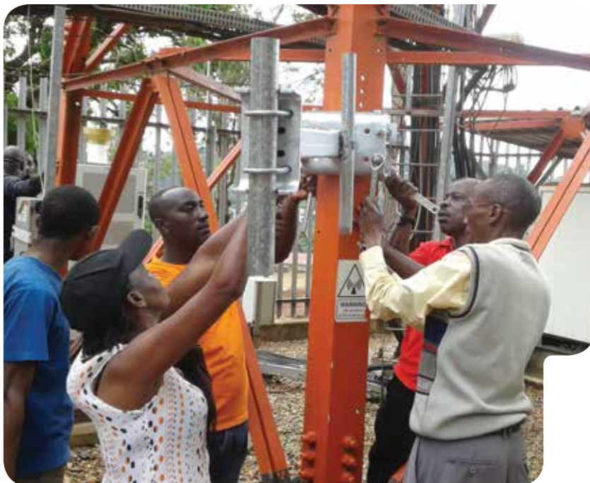
AWS BEING PREPPED FOR DEPLOYMENT ON A CELL TOWER IN UGANDA. A LIGHTNING SENSOR WILL ALSO BE DEPLOYED ON THIS TOWER. TO INCREASE THE LIKELIHOOD THAT EACH LIGHTNING STRIKE IS PROPERLY LOCATED, THE LIGHTNING LOCATING SYSTEM WILL ALSO INTEGRATE LIGHTNING DATA FROM NEIGHBOURING NETWORKS IN BURUNDI, KENYA AND TANZANIA, MAKING FOR IMPROVED REGIONAL COOPERATION IN EARLY WARNING SYSTEMS. PHOTO BY SOLOMON MANGENI.
