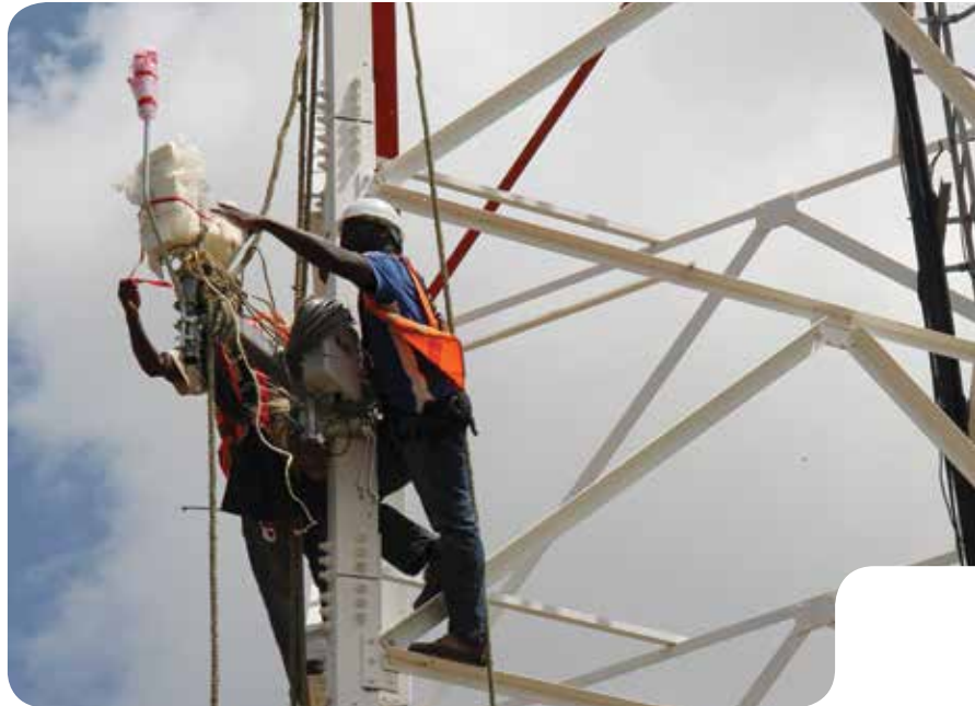
AN ALL-IN-ONE AUTOMATIC WEATHER STATION (AWS) BEING INSTALLED ON A CELL-PHONE TOWER NEAR KOTIDO, UGANDA. FIVE SUCH AWS HAVE BEEN INSTALLED ON CELL TOWERS ACROSS UGANDA THROUGH THE COUNTRY'S STRENGTHENING CLIMATE INFORMATION AND EARLY WARNING SYSTEMS PROJECT. CONNECTED DIRECTLY INTO THE TELEPHONE BACKBONE NETWORK, THE DATA ARE SENT TO UGANDA NATIONAL METEOROLOGICAL AUTHORITY (UNMA) FOR PROCESSING AND ANALYSIS. THE FIVE STATIONS, EACH OF WHICH ALSO INCLUDE A LIGHTNING LOCATING SENSOR, WILL PROVIDE DATA TO AN END-TO-END MONITORING AND FORECASTING SYSTEM, WHICH ALLOWS UNMA TO ISSUE EARLY WARNINGS FOR IMPENDING HAZARDOUS THUNDERSTORMS, CONNECT WITH REGIONAL MONITORING SYSTEMS AND IMPROVE THE COUNTRY'S OVERALL SUSTAINABILITY OF INVESTMENTS IN CLIMATE INFORMATION SERVICES. PHOTO BY SOLOMON MANGENI.
