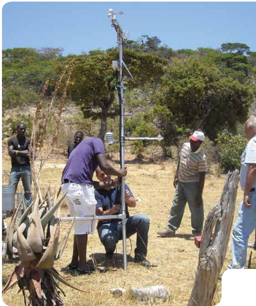
INSTALLING IMPROVED WEATHER MONITORING TECHNOLOGY IS THE FIRST STEP TO CREATING AN INCLUSIVE END-TO-END SYSTEMATIC APPROACH.
