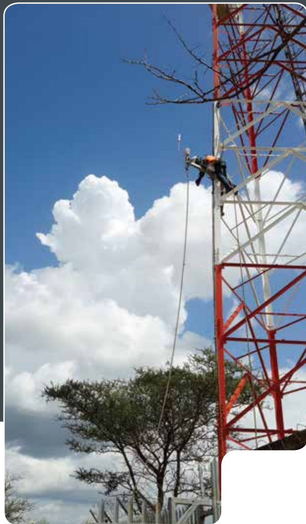
DEPLOYING AN ALL-IN-ONE AWS ON A CELL TOWER.
