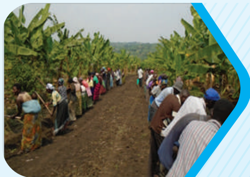
Communities working together to construct roads in Bunyangabu District. The Inclusive and Sustainable New Communities (ISNC) project was implemented with support from the Republic of Korea. This is an example of values-based approaches to community level development
