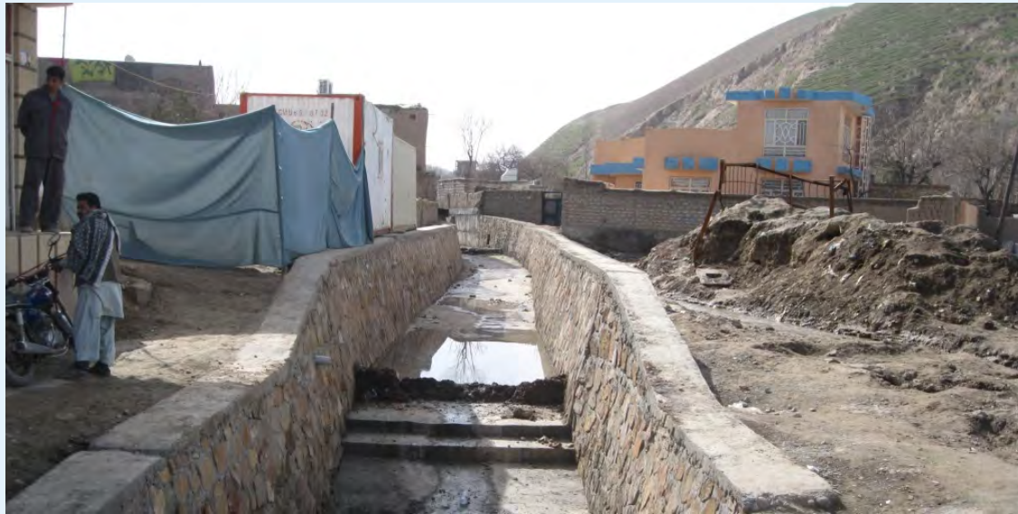
This repaired canal will protect Qala-e-Naw city from flash-floods in the coming spring season.
