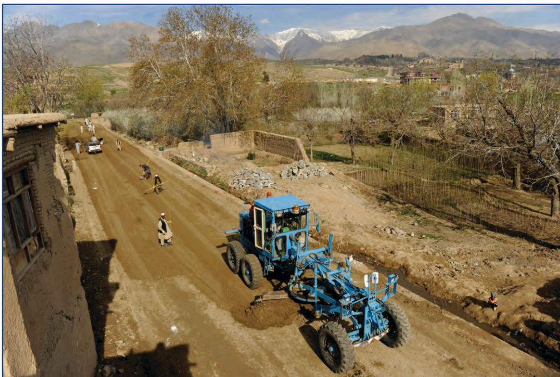
A new road constructed under NABDP makes travelling safer and connects communities.
