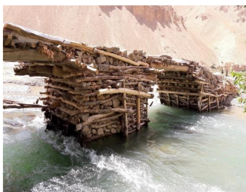
Figure 1: Temporary rehabilitation of Dahne sia Dara Bridge in Yaka wulung No. 2 district – (Bamyan)
