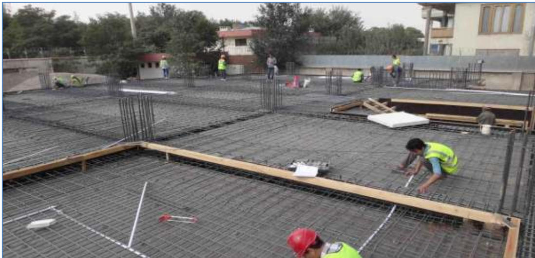
Photo 4: Work in progress for the formworks and reinforcement of the basement floor slab. Photo Credit: MoI.
