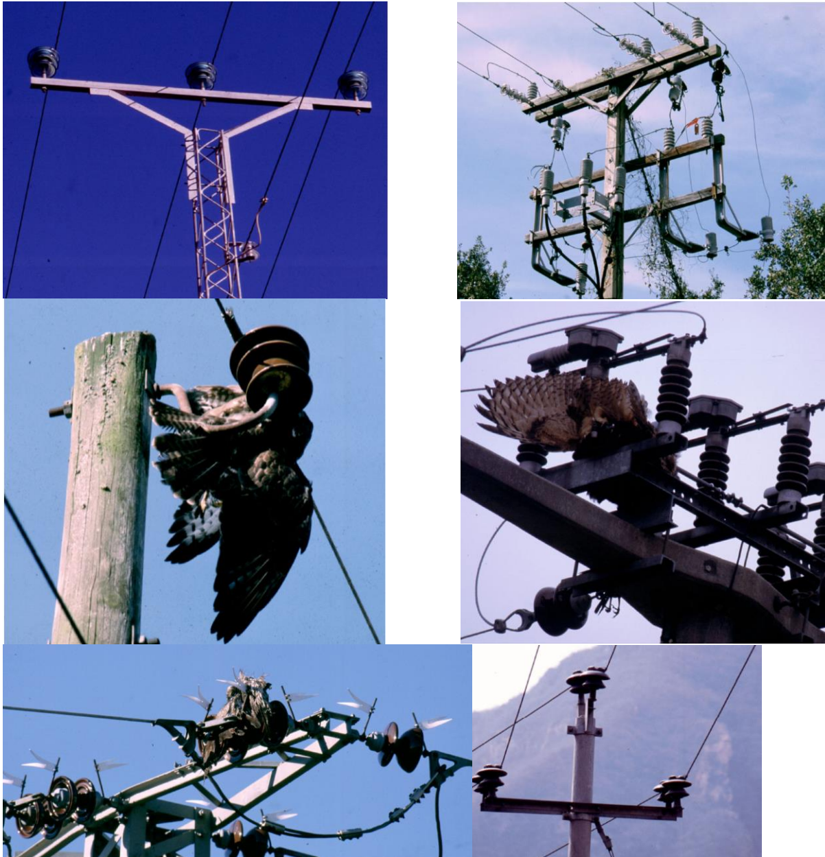
Figure 45 Typical designs of poles causing high bird mortality by electrocution 99
