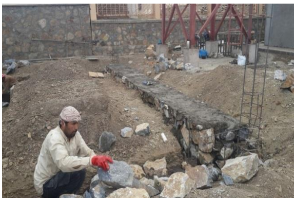
Generator shelter at Bamyan
