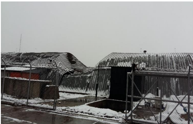
Warehouse 3 collapsed and need to be replaced
