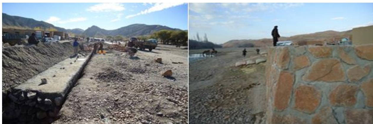
SGP project for retaining wall in Gulchin village of Qadis district, Badghis Province under construction and completed later in 2015.
