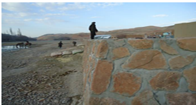
Retaining wall project completed in Gulchin village of Qadis district, Badghis Province
