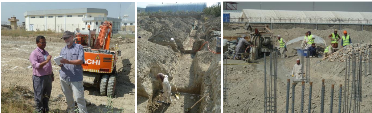
Figure 12, 13, and 14: Construction and building foundation work of the IEC Education Center in its Kabul Compound. (Photo Credit: UNDP)
