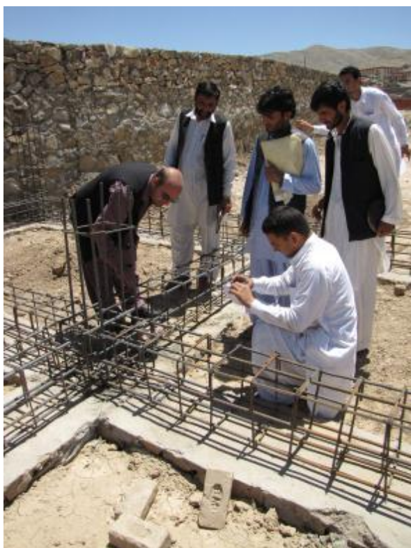
Figure 6: ELECT II and IEC engineers conducting quality control inspection in Wardak. Credit: UNDP
