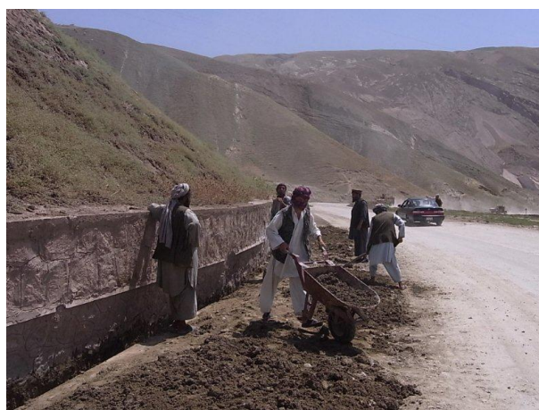
Figure 10: Reintegrees work on maintenance of road damaged by flood in Kunduz province. (Photo credit: UNDP)
