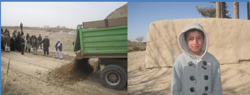
Figures 5 and 6: Reintegrees and community members working on a road project (left), and a local child expresses his appreciation for the road construction. “We are happy. We can bring vehicles up to our village when we purchase goods.” (Photo credit: UNDP)
