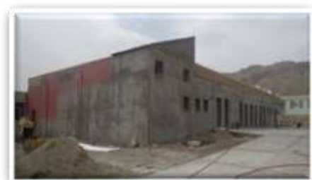
Figure 5: View of the construction of the RTA Herat Building, being monitored by ASGP LoA staff. Photo Credit: ASGP
