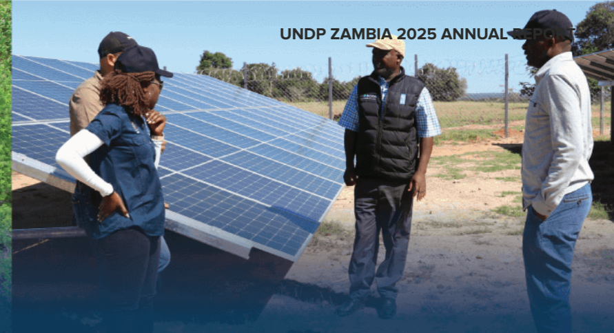
Through the Smart Health Systems project, Sekelela Health Post is receiving solar power at approximately 3 kiloWatt-peak delivered through five solar photovoltaic panels, alongside a satellite connectivity system.
