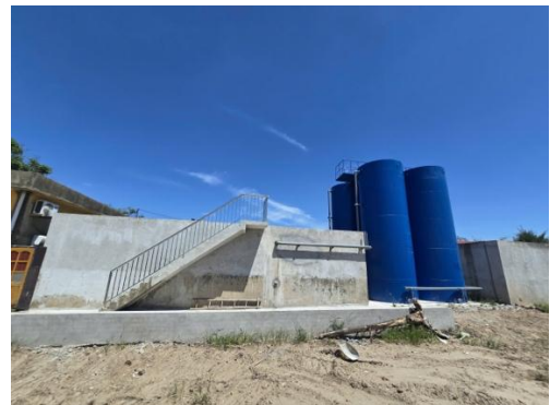
Picture 10. Wastewater treatment plant in in Ninh Co Fishing Port
