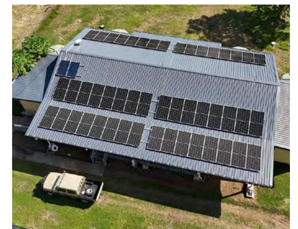
The solar system at the Innovation Hub in Buka
