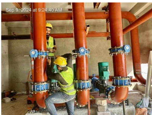
Chiller rooms Mechanical piping, Oncology and Nuclear Medicine Hospital, Al-Shifaa Complex, Nineveh Governorate, September 2024
