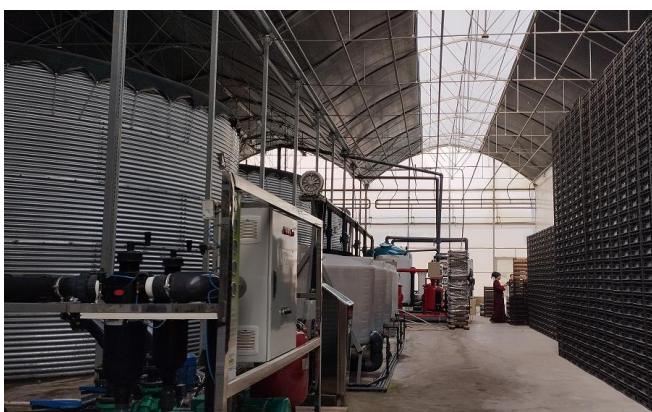
Photo 9. Reverse osmosis facilities
