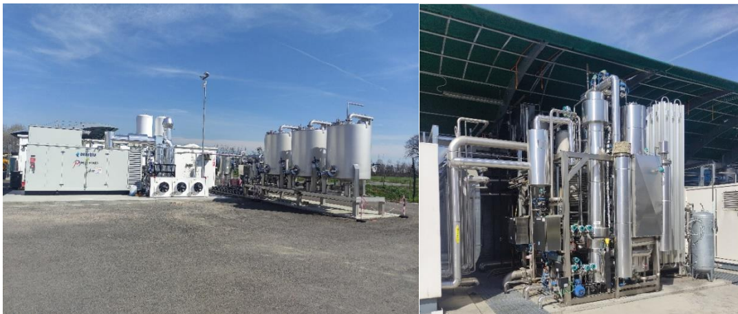
Figure 6: Part of the plant for biogas purification to liquefied biomethane \text{H}_2\text{S} removal and drying (on the left), cryogenic cooling for \text{CO}_2 separation (on the right)
